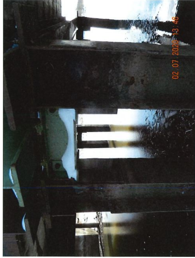
TYPICAL HEAVY RUST OF H-PILES
