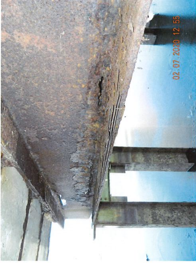
SECTION LOSS OF WEST BENT CAP BEAM AT BENT 3
