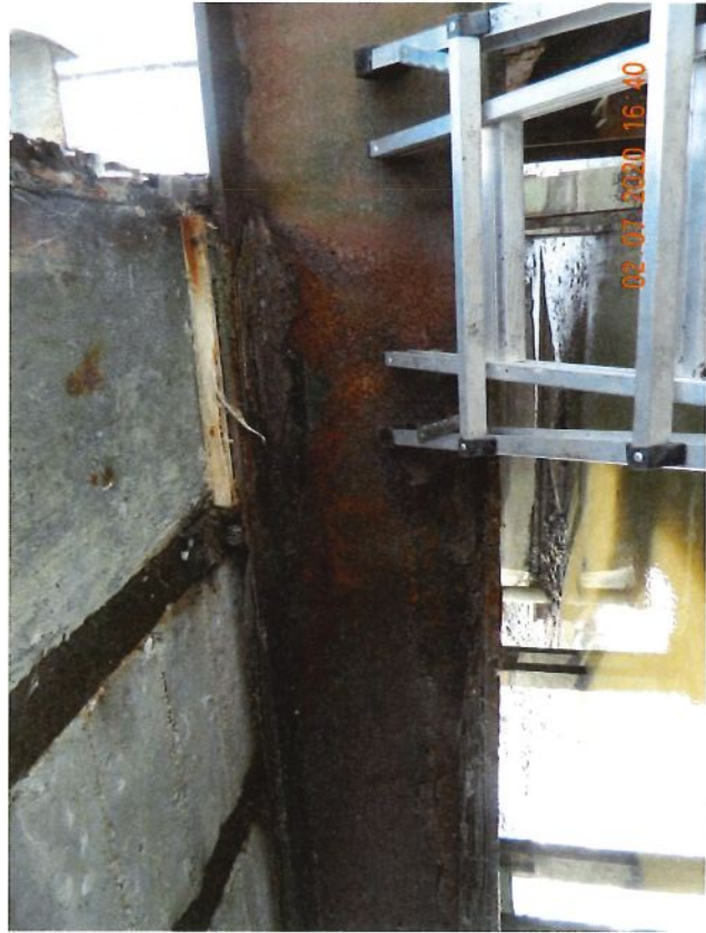
SECTION LOSS OF EAST BENT CAP BEAM AT BENT 5
