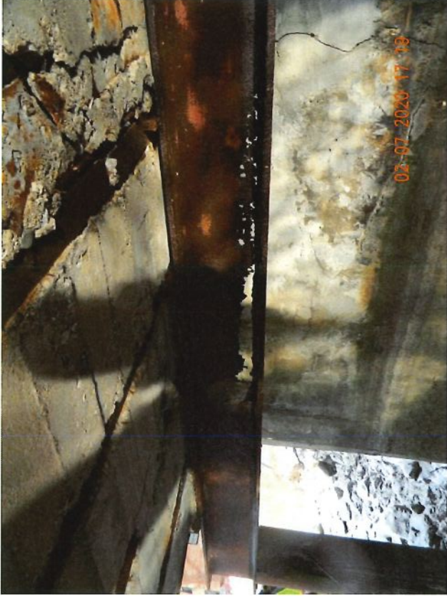
SECTION LOSS OF CAP BEAM AT BENT 6
