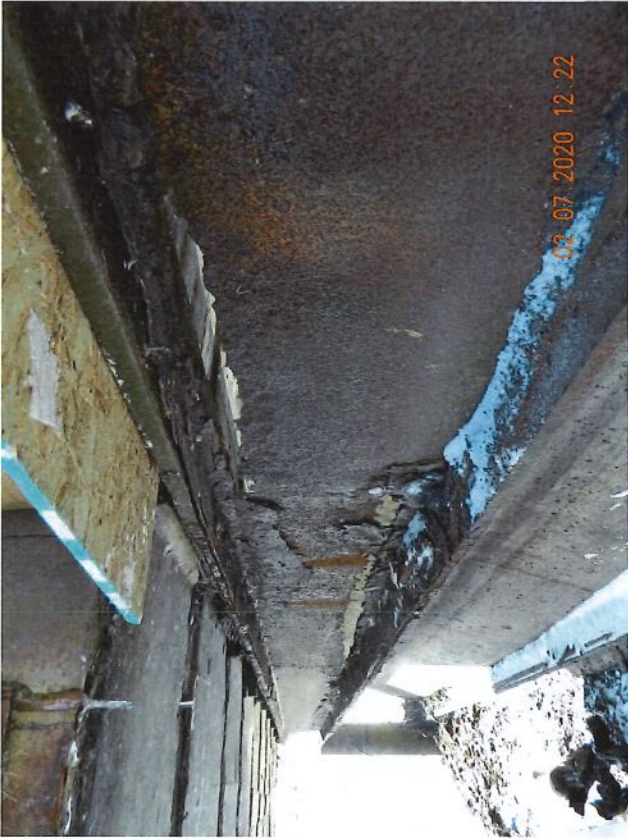
SECTION LOSS OF CAP BEAM AT BENT 2
