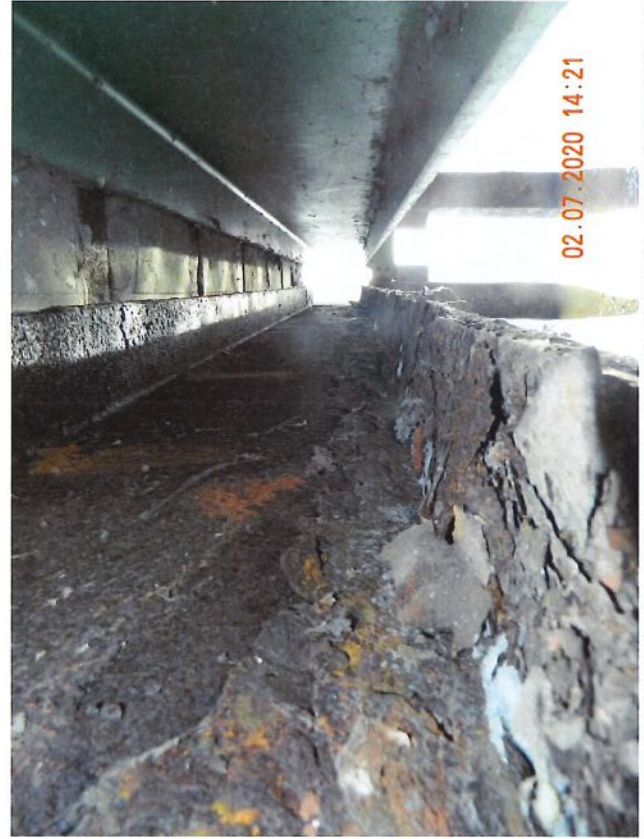
TYP. PACK RUST IN ORIGINAL BENT CAPS AT BENTS 3, 4 & 5
