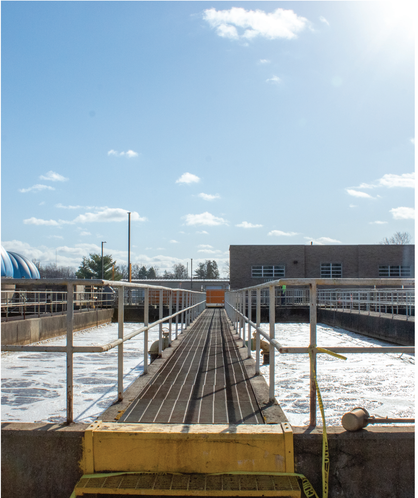
WASTEWATER TREATMENT PLANT
