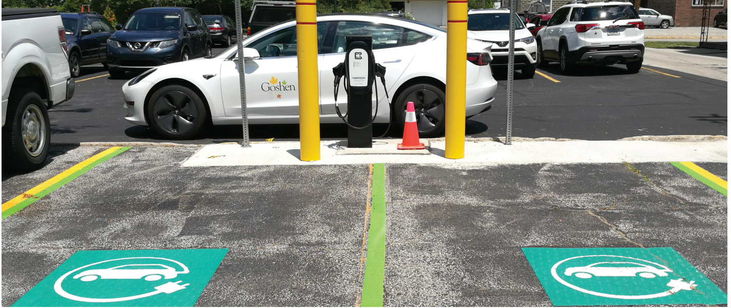
CITY OF GOSHEN PUBLIC EV CHARGING STATION
