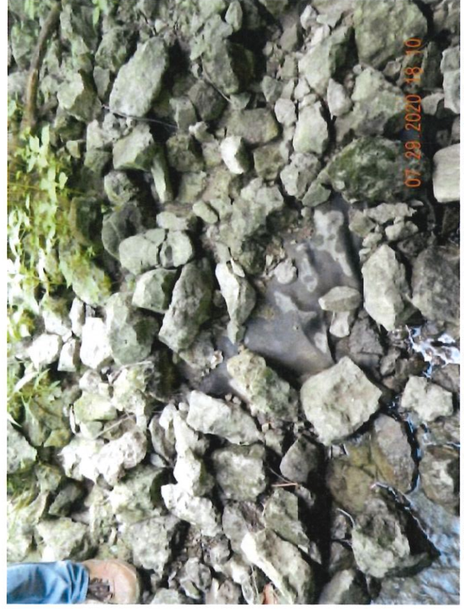
EXPOSED GEOTEXTILES AT WEST SPILL SLOPE
