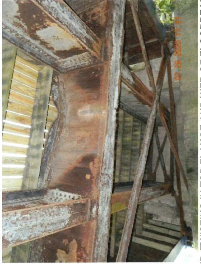
TYP. TWISTING IN TOP FLANGE AND WEB OF FLOORBEAMS
