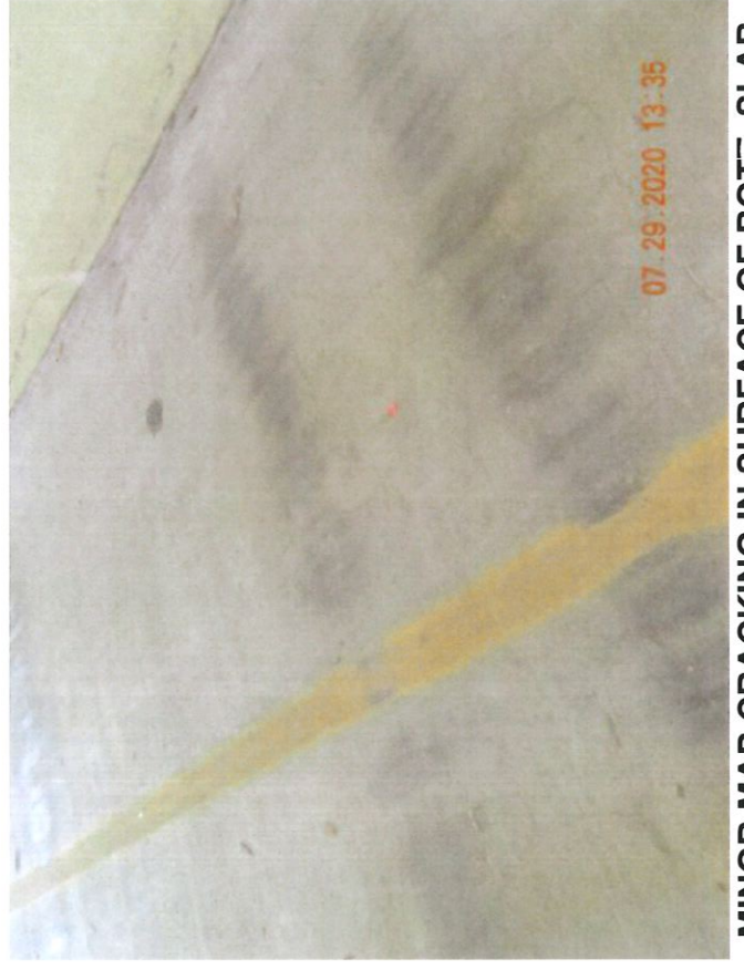
MINOR MAP CRACKING IN SURFACE OF BOT™ SLAB
