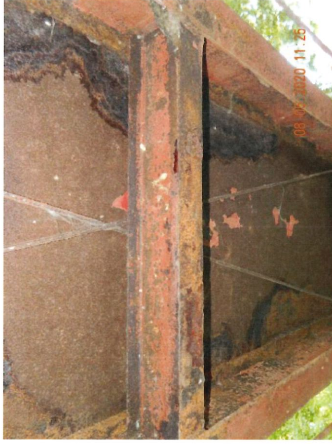
HEAVY RUST IN STEEL DIAPHRAGM
