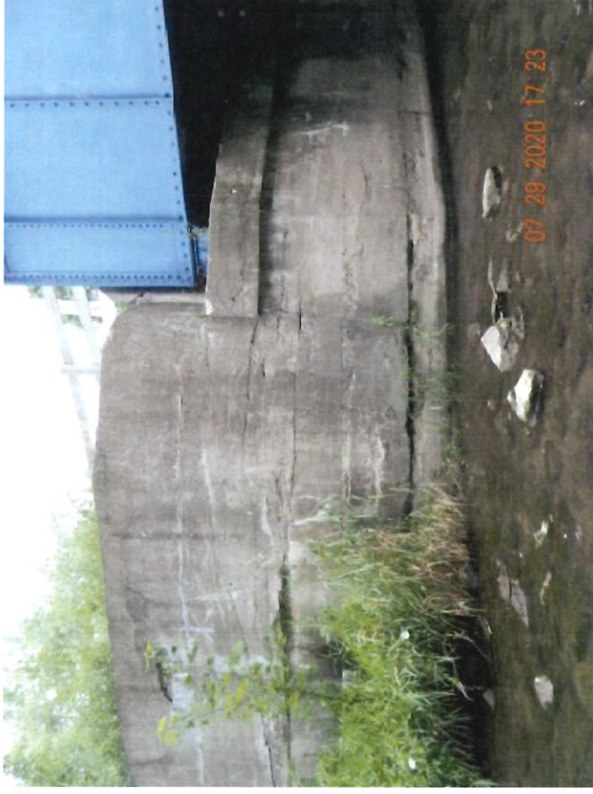
SCALING AND ABRASION IN EAST ABUTMENT
