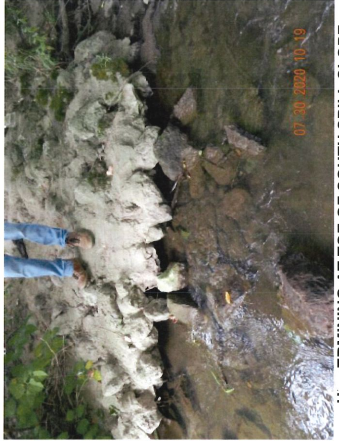
UNDERMINING AT TOE OF SOUTH SPILL SLOPE
