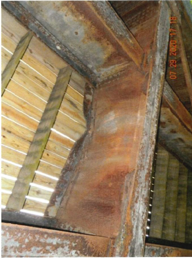
TYP. TWISTING IN TOP FLANGE AND WEB OF FLOORBEAMS
