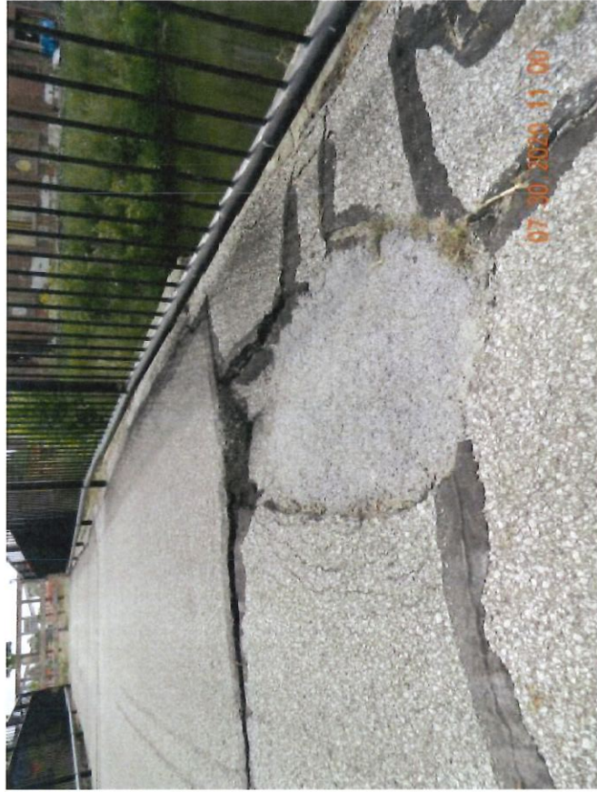
SETTLEMENT IN WEST APPROACH
