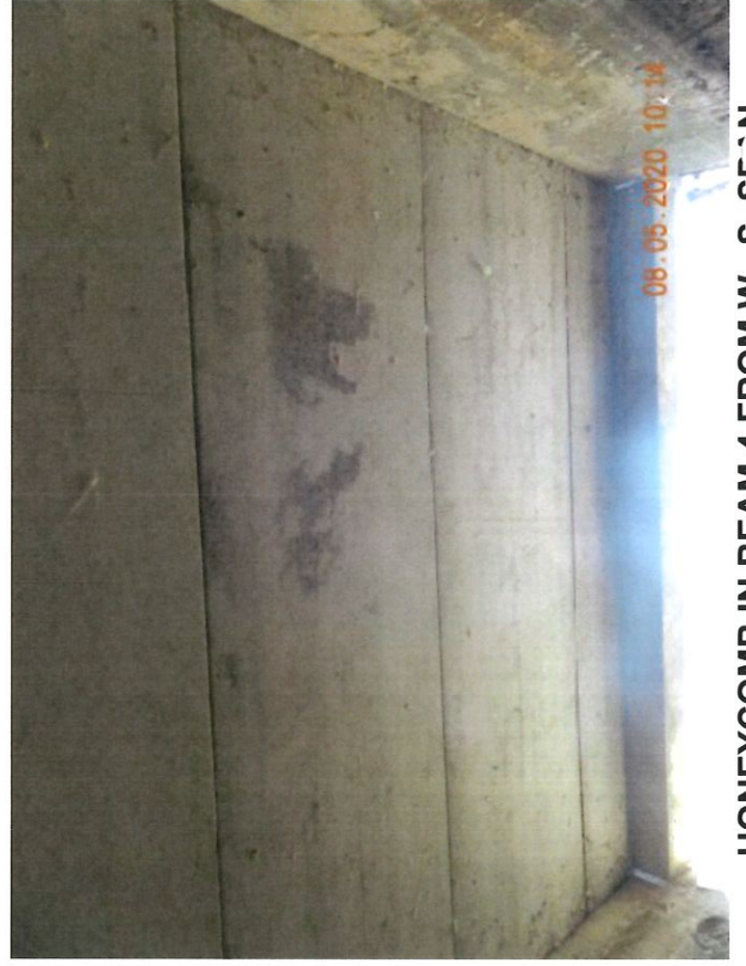
HONEYCOMB IN BEAM 4 FROM W., S. SPAN
