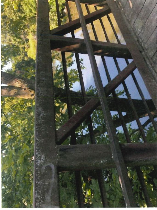
TREE NEXT TO SOUTH TRUSS KEEPING BRIDGE WET
