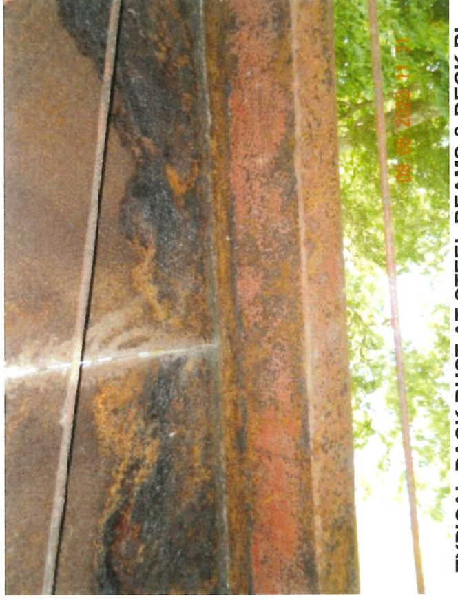
TYPICAL PACK RUST AT STEEL BEAMS & DECK PL
