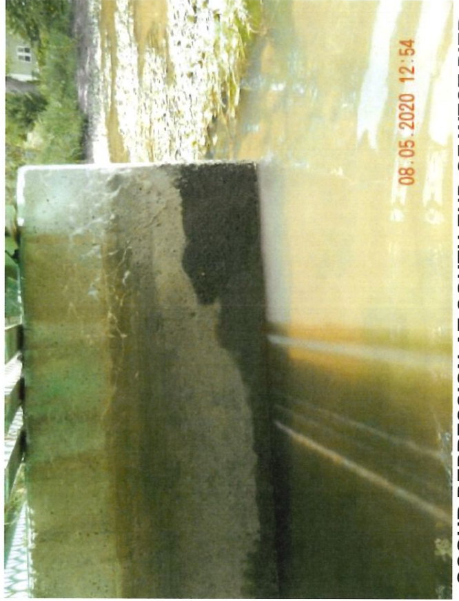
SCOUR DEPRESSION AT SOUTH END OF WEST PIER
