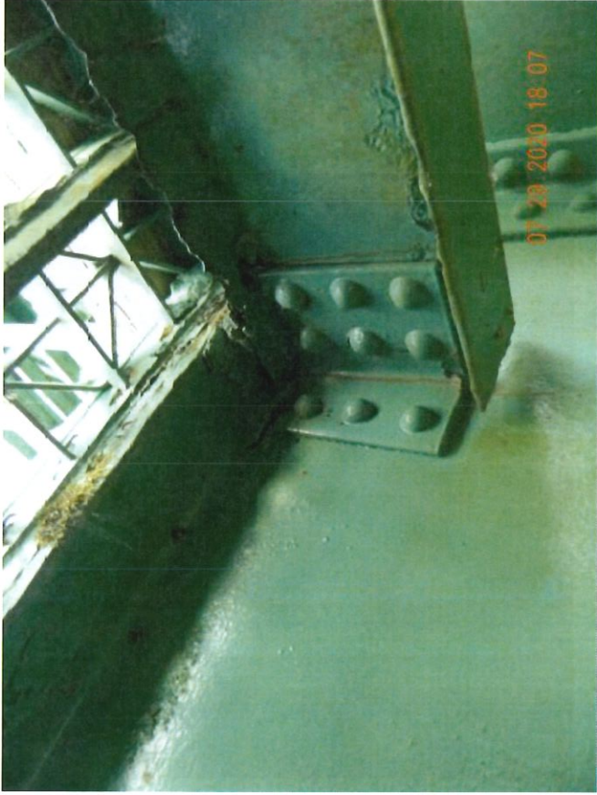
TYP. SECTION LOSS AT TOP FLANGE OF STRINGER/ FB CONN.
