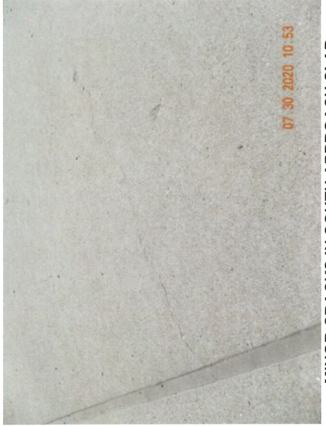
MINOR CRACKS IN SOUTH APPROACH SLAB
