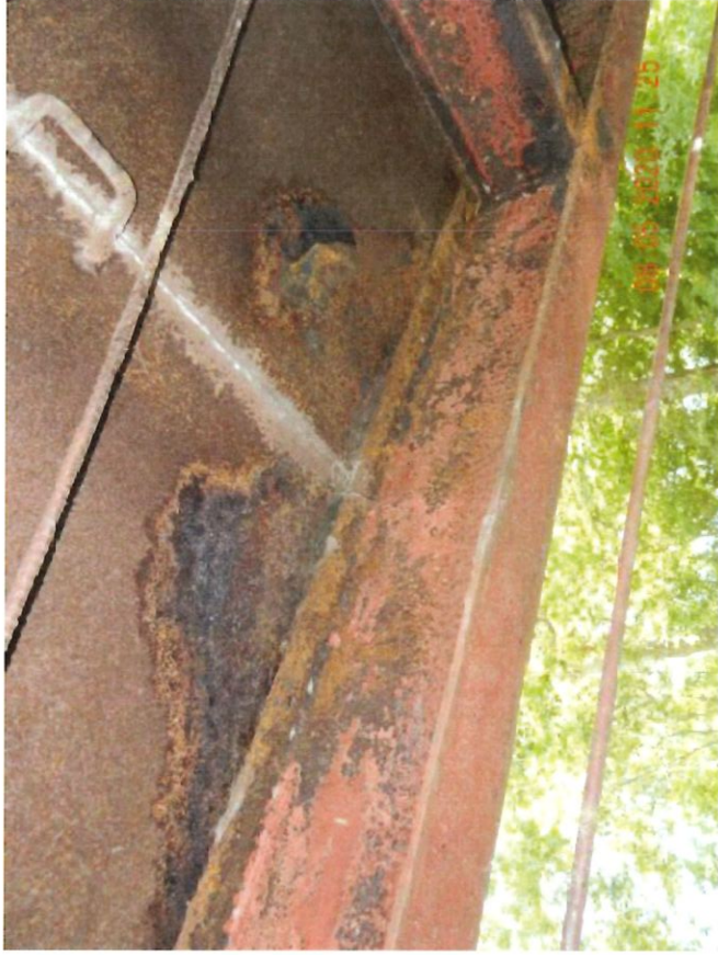
TYPICAL RUST & PITTING OF STEEL BEAMS AND DECK PL
