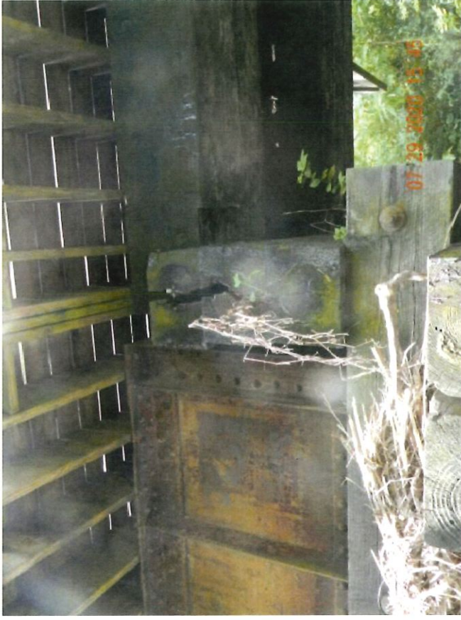
LARGE SPLIT IN TIMBER CAP OF EAST PIER OF MAIN SPAN
