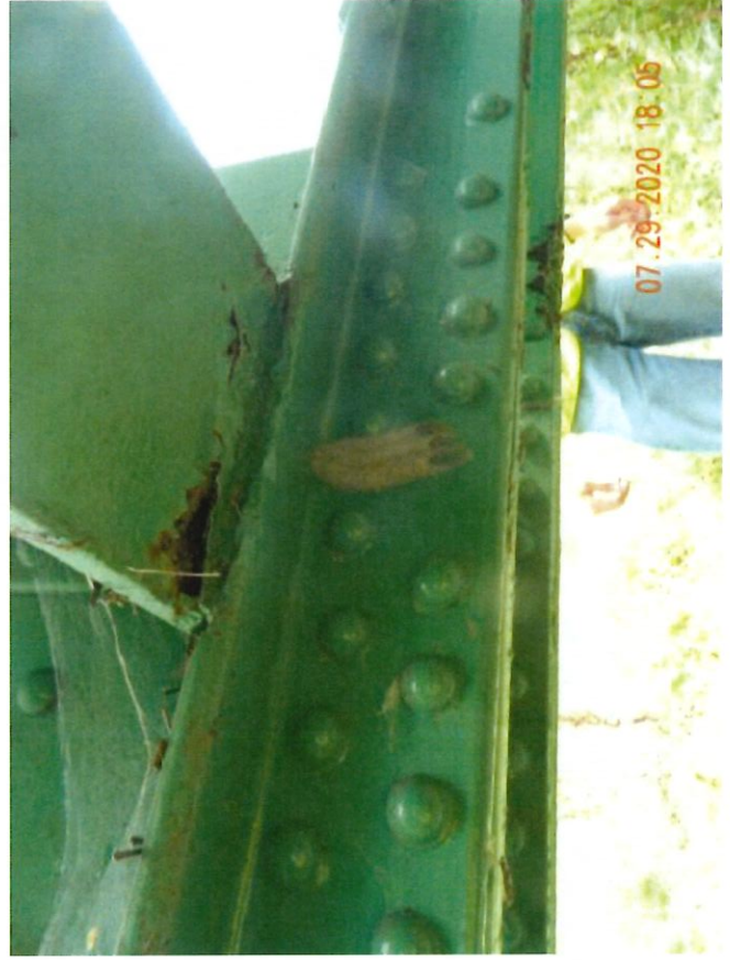
TYP. PACK RUST AT FLOORBEAM TO LOWER CHORD CONN.
