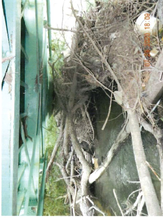
DEBRIS UNDER BRIDGE AND BETWEEN LATERALS
