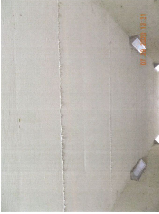
UNDERSIDE OF TOP SLAB W/ LONGITUDINAL CRACKING
