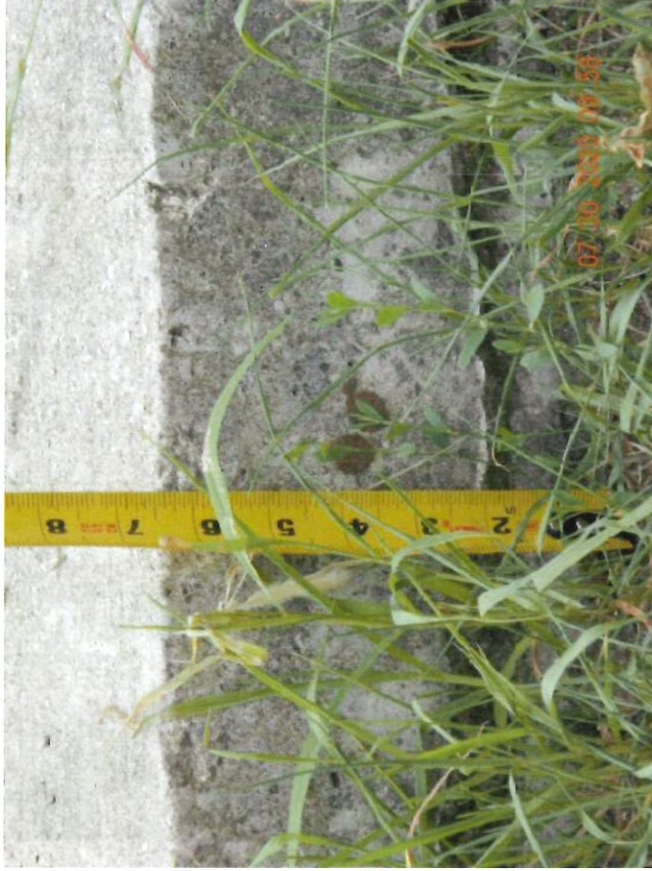
6.5" DROP OFF AT NORTH APPROACH
