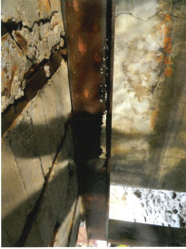
SECTION LOSS OF CAP BEAM AT BENT 6
