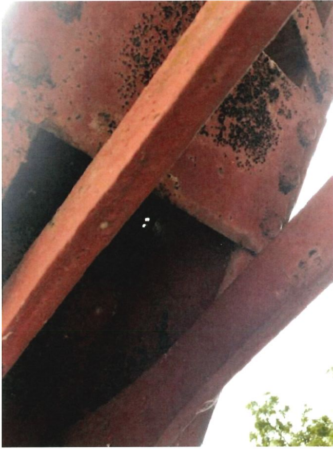
PITTING AND MINOR SECTION LOSS AT UPPER CHORD
