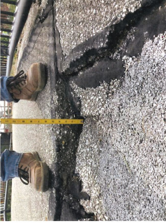
SETTLEMENT IN WEST APPROACH
