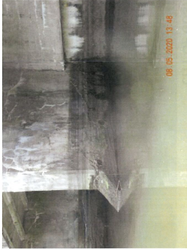
TYP. SCALING BELOW THE WATERLINE
