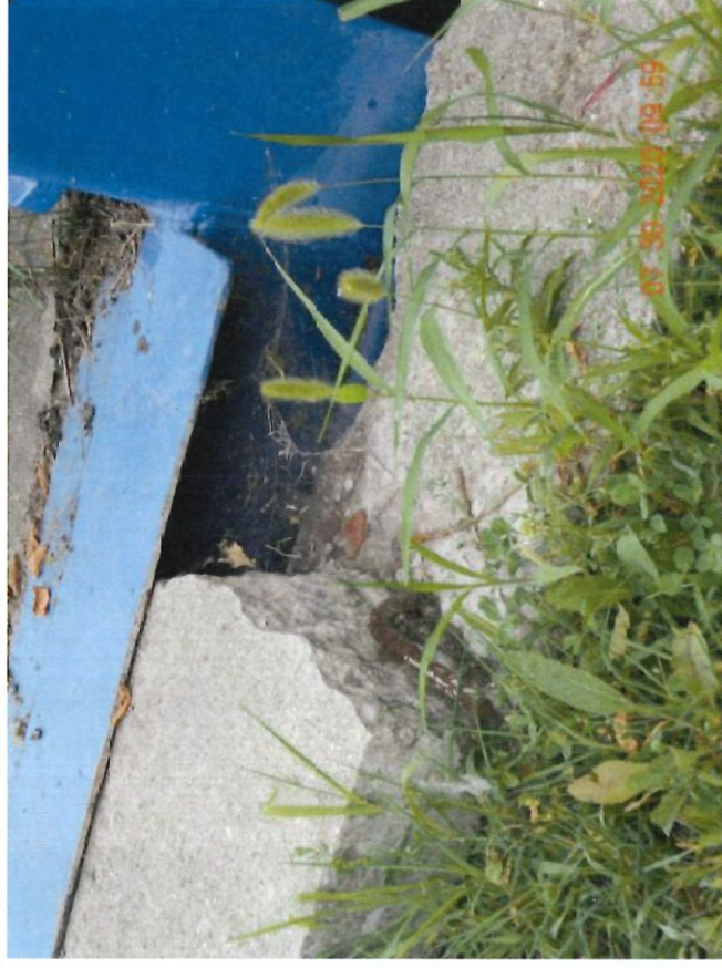
SPALL IN WEST CORNER OF NORTH END BENT MUDWALL
