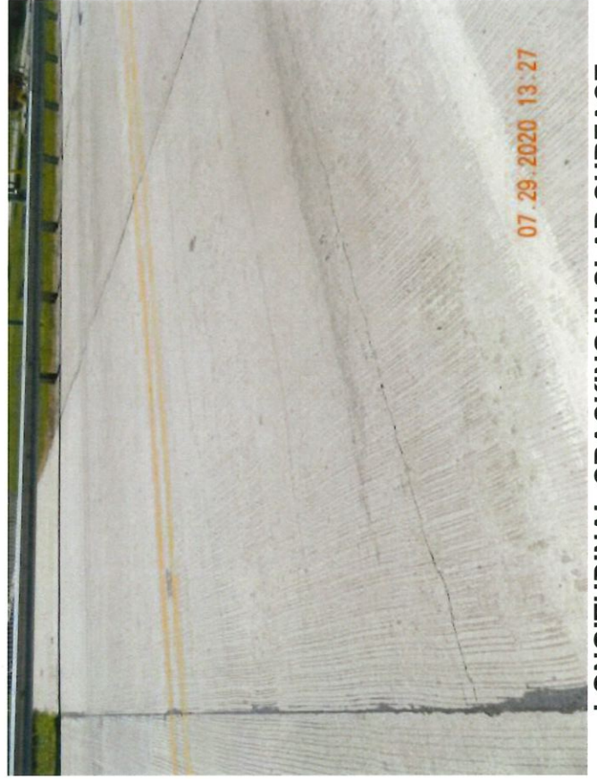
LONGITUDINAL CRACKING IN SLAB SURFACE
