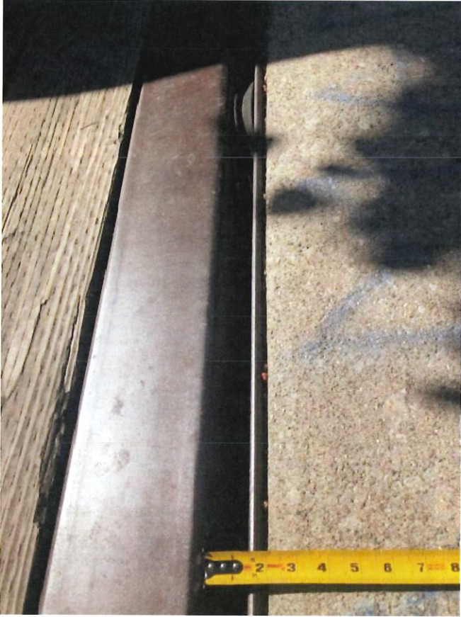
EXPANSION JOINT AT WEST END MISSING MATERIAL
