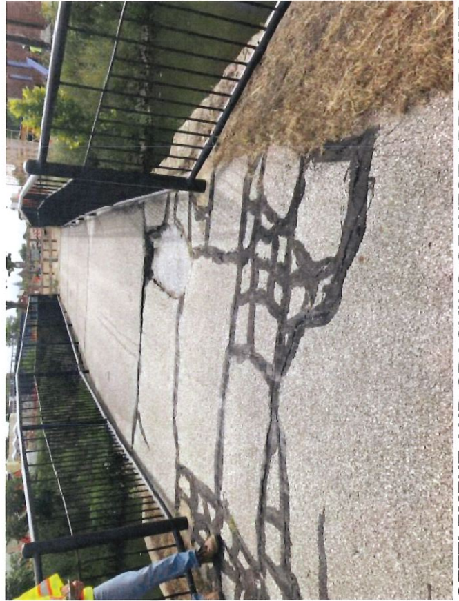
SETTLEMENT AND CRACKING OF WEST APPR. PAVMT.
