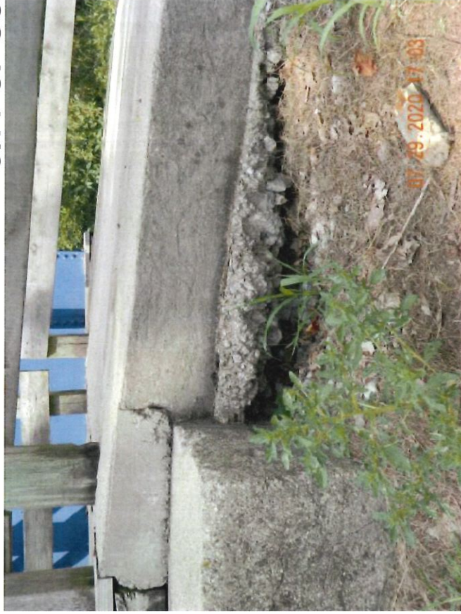
UNDERMINING IN EAST APPROACH
