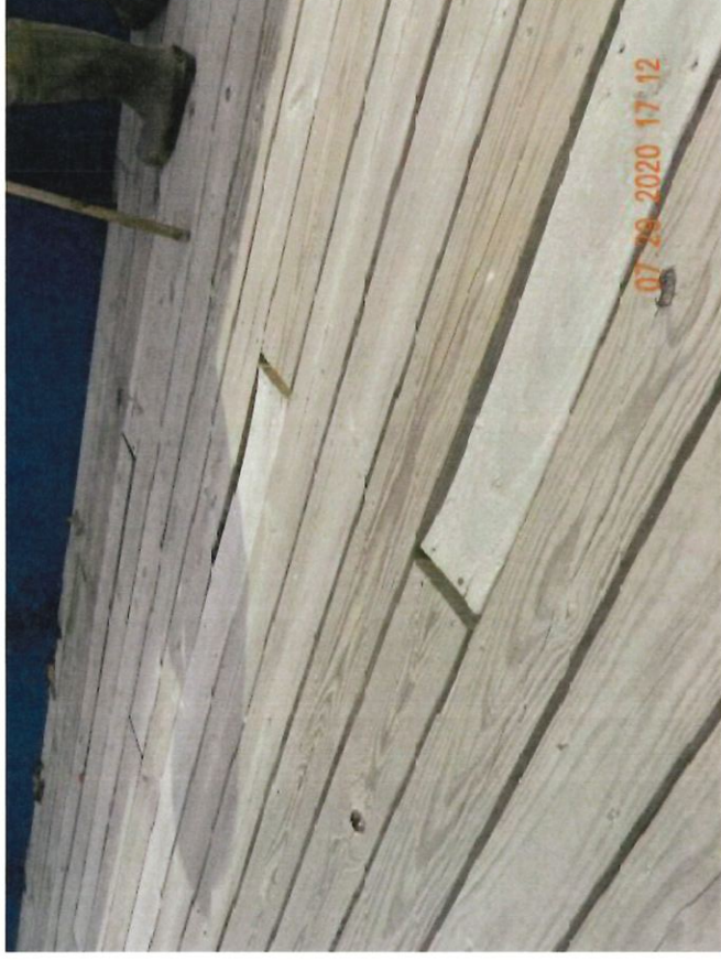
WARPING IN DECK TIMBER BOARDS
