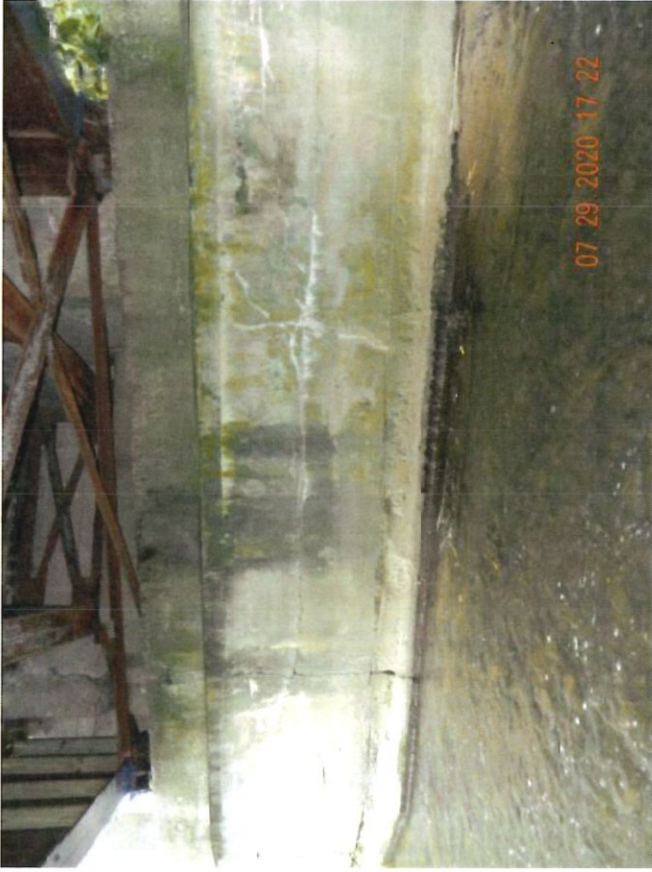
CRACKING AND SCALING IN WEST ABUTMENT
