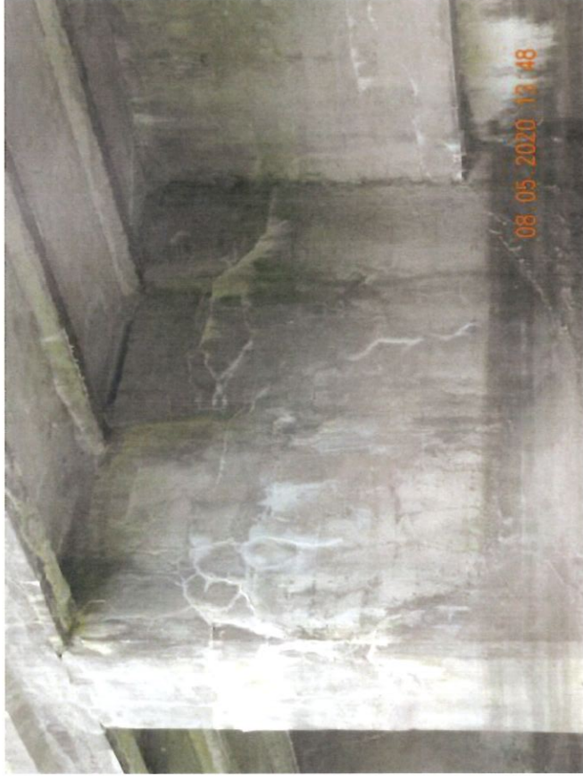
HEAVY CRACKING WITH LEACHING IN WEST PIER
