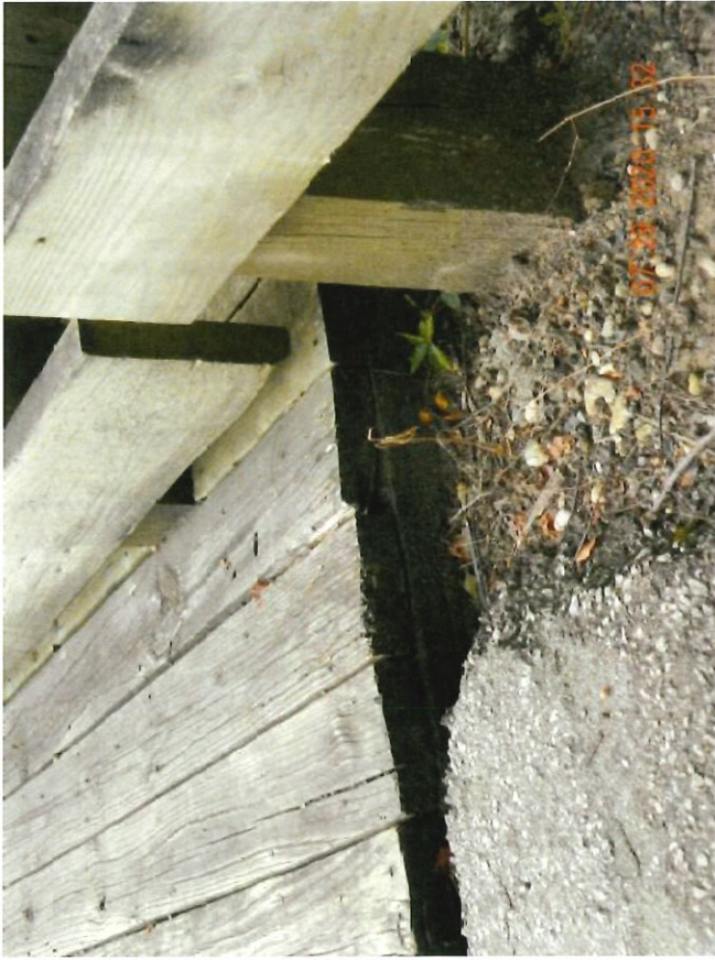
EROSION BEHIND SOUTHWEST CORNER
