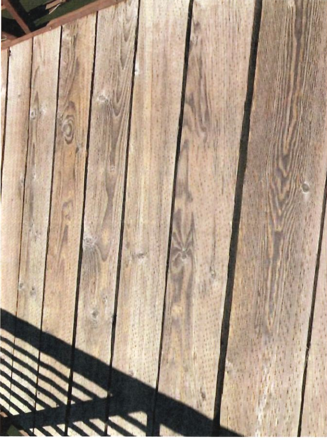
SEPARATION OF TIMBER BOARDS
