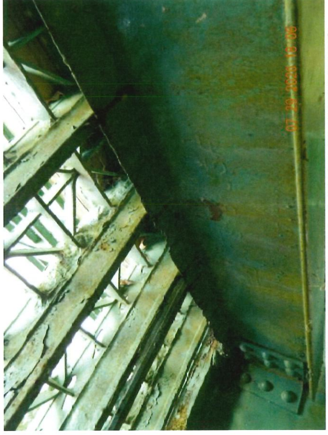
SECTION LOSS IN TOP FLANGE OF STRINGERS
