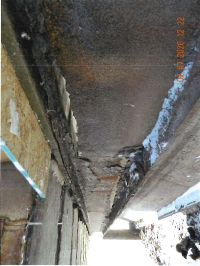
SECTION LOSS OF CAP BEAM AT BENT 2
