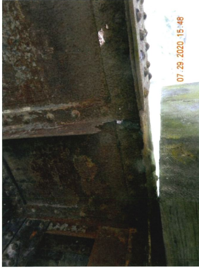
100% SECTION LOSS IN STEEL STIFFENERS
