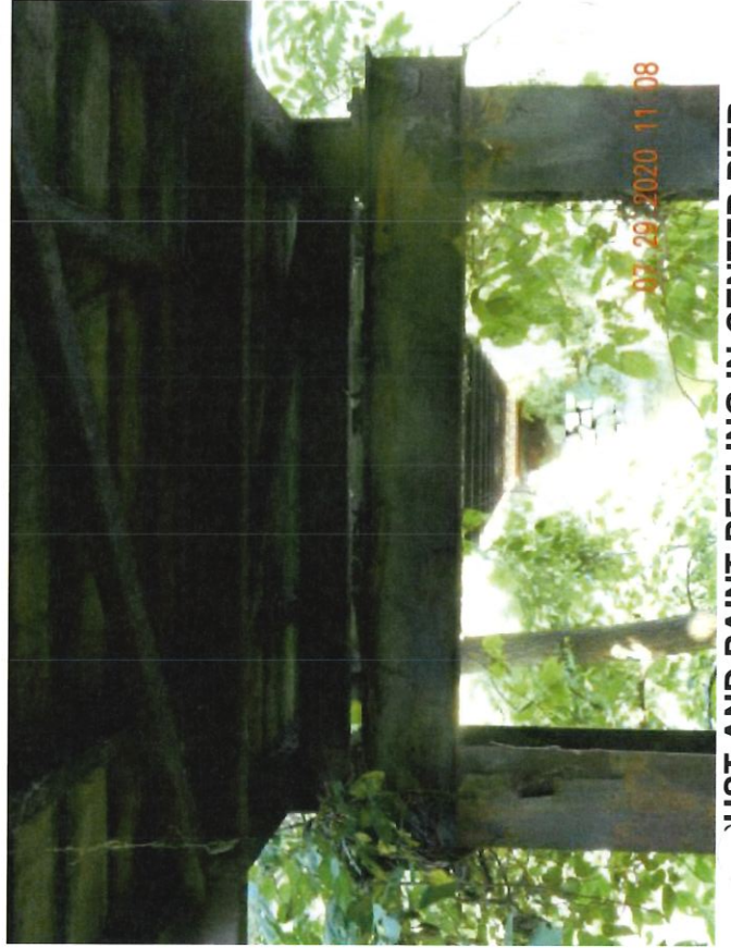
RUST AND PAINT PEELING IN CENTER PIER
