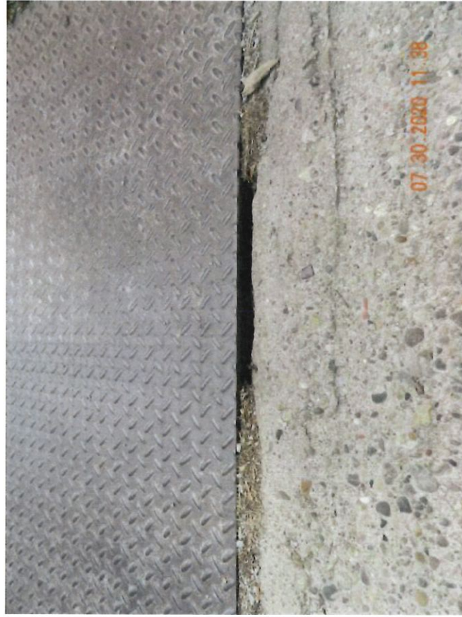
GAP AT WEST APPROACH END OF BRIDGE
