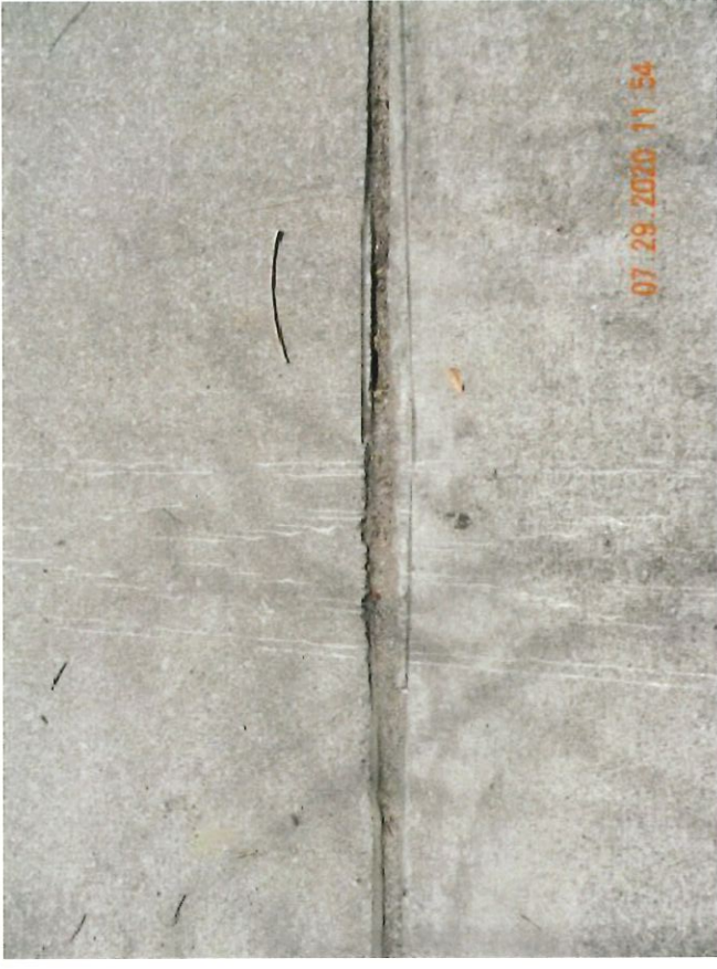
FAILED WEST EXPANSION JOINT DECK
