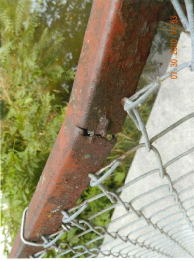
BROKEN TOP BAR IN BENT RAIL AT WEST END
