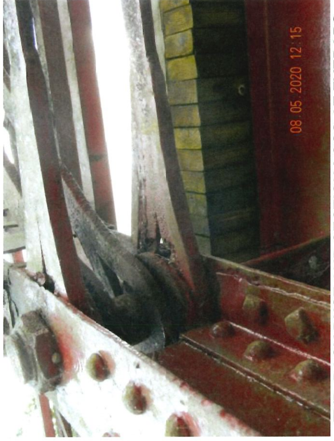
TYP. PACK RUST AND SECTION LOSS AT EYEBARS
