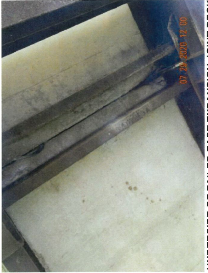
UNDERSIDE OF FAILED EAST EXPANSION JOINT DECK
