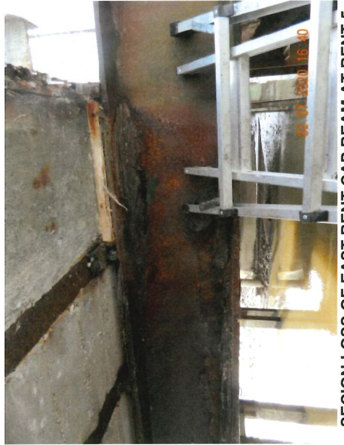
SECTION LOSS OF EAST BENT CAP BEAM AT BENT 5
