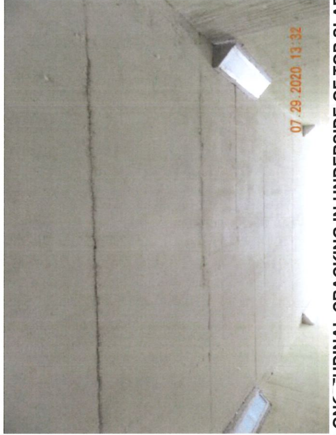
LONGITUDINAL CRACKING IN UNDERSIDE OF TOP SLAB
