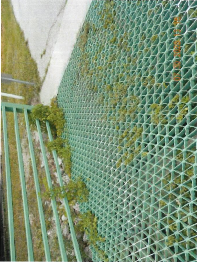
VEGETATION GROWING UNDER EAST END OF BRIDGE
