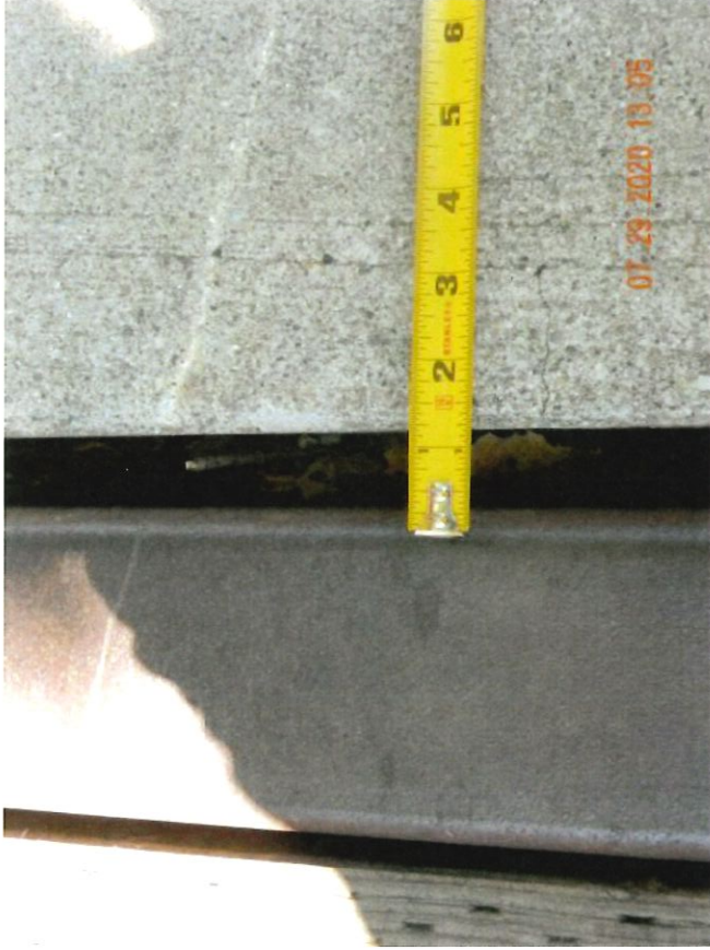
>1" SEPARATION AT EAST APPROACH END
