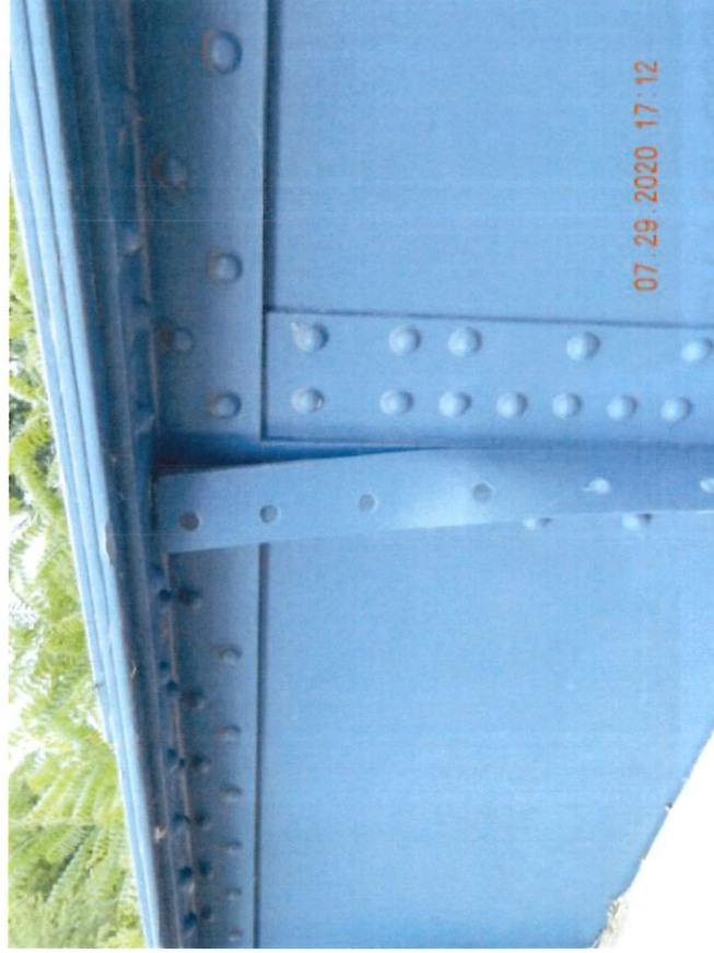
TWISTED STEEL STIFFENER ABOVE DECK
