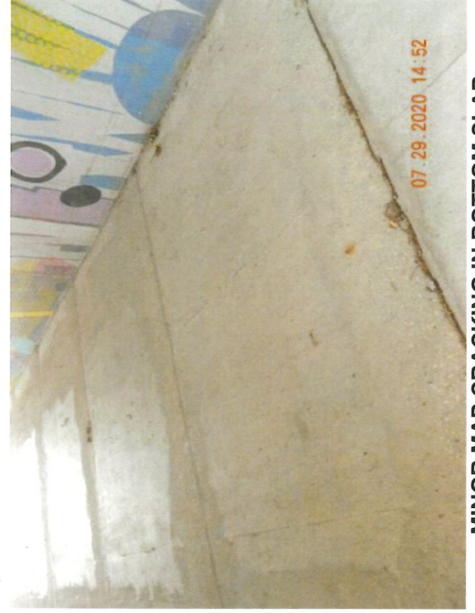
MINOR MAP CRACKING IN BOTTOM SLAB
