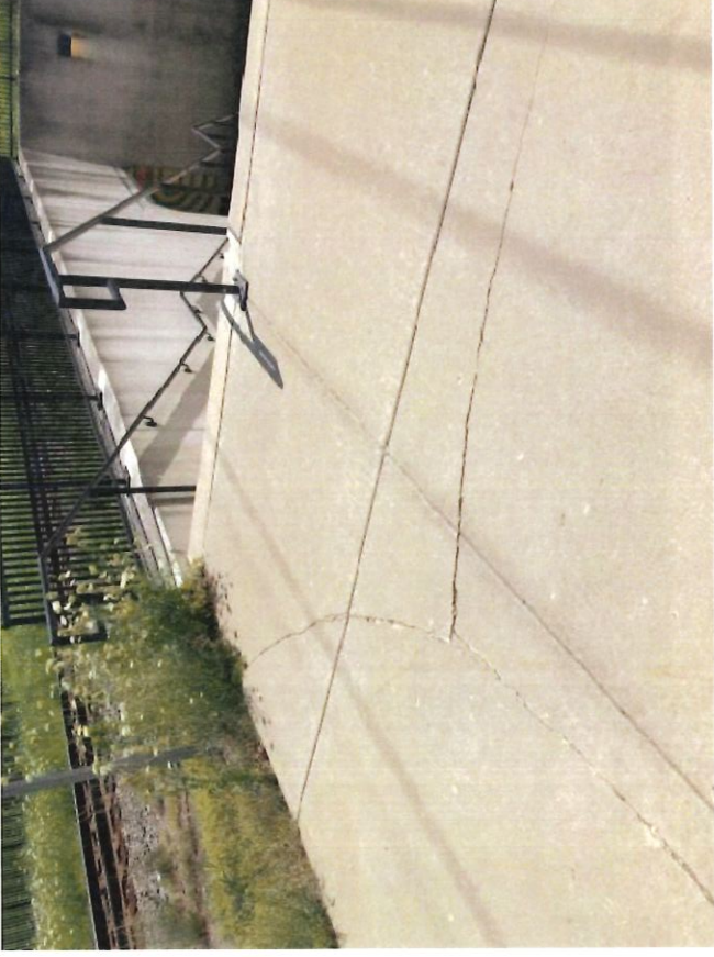
CRACKING IN SIDEWALK APPROACH AT WEST STAIRS
