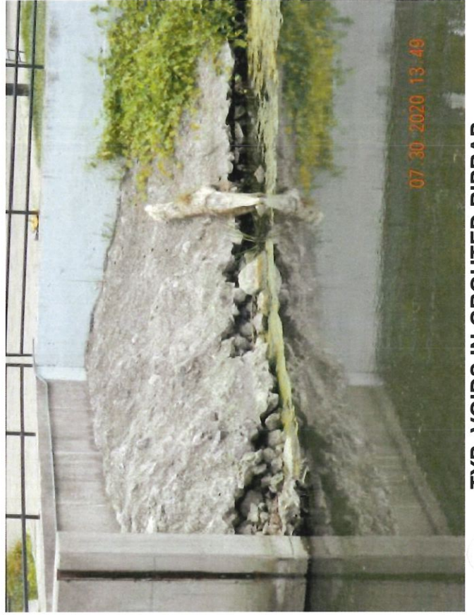
TYP. VOIDS IN GROUTED RIPRAP
