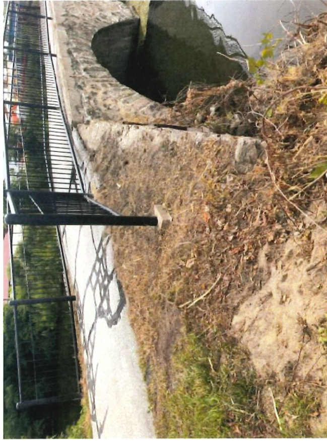
EROSION AT SOUTHWEST WINGWALL
