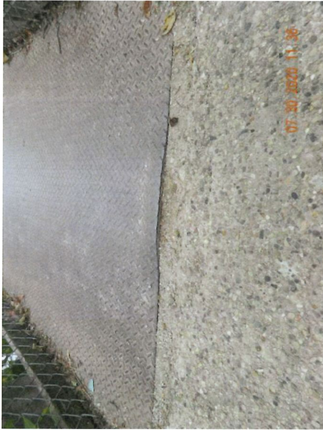
DENT IN DECK PLATE AT EAST END
