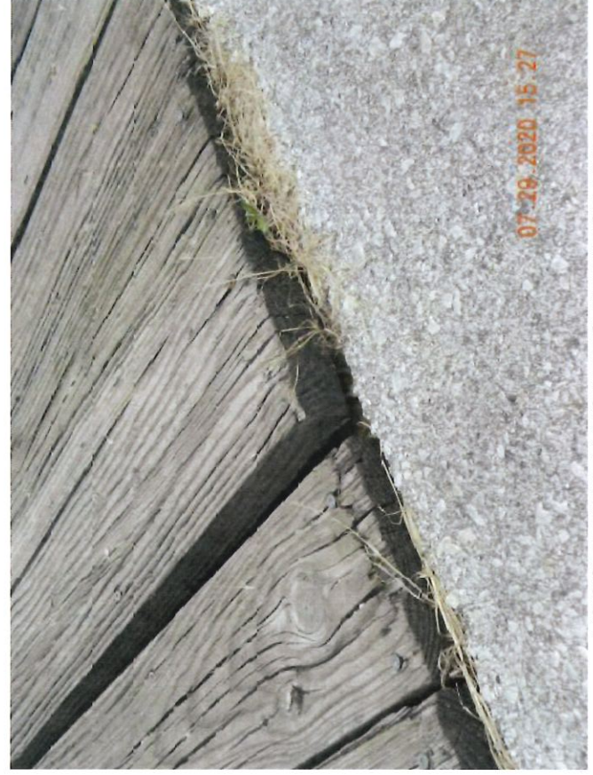
LOOSE TIMBER BOARDS AT WEST END
