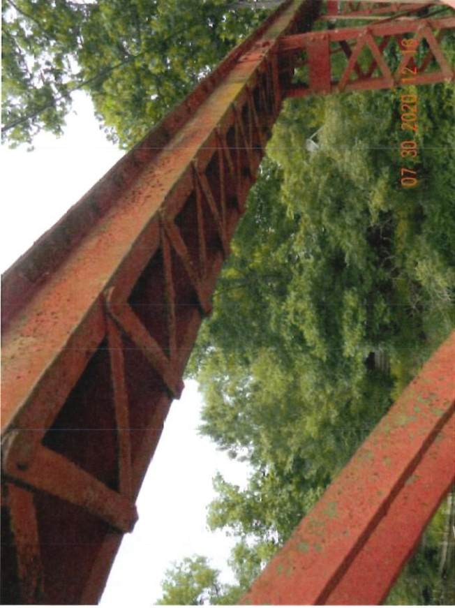
TYP. PITTING AND PAINT PEELING OF TRUSS
