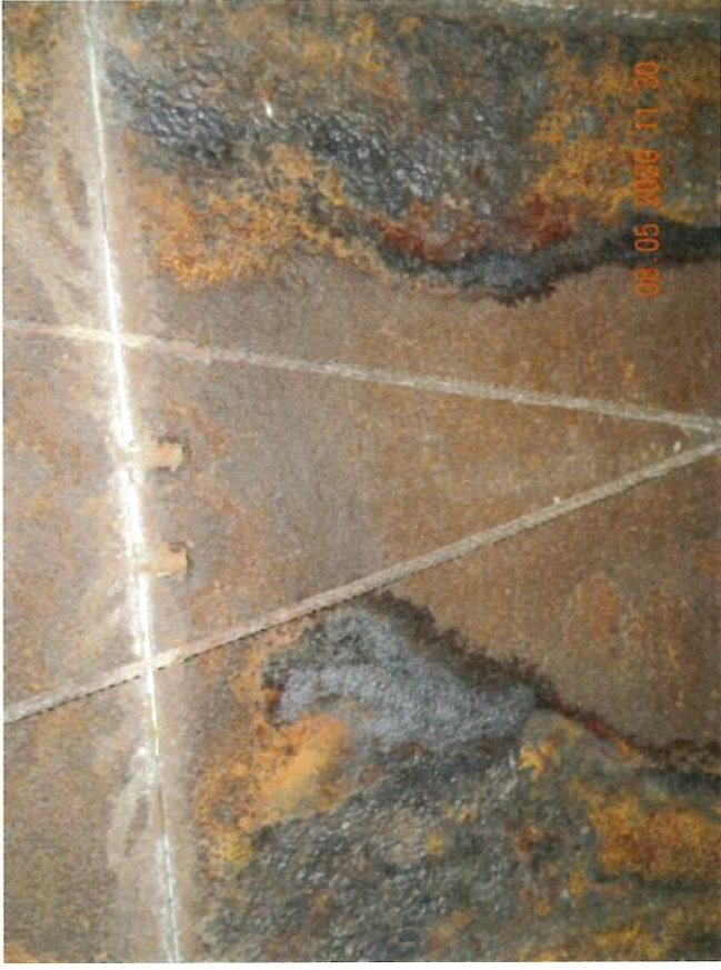
RUST AND SEPARATION OF DECK PL NEAR MIDSPAN
