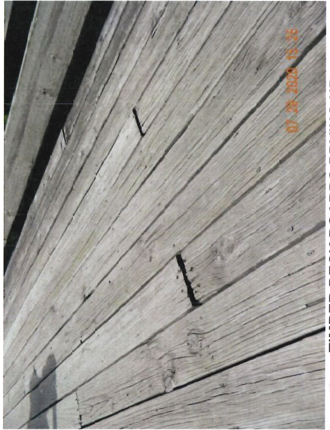
TIMBER DECK BOARDS PRYING UP
