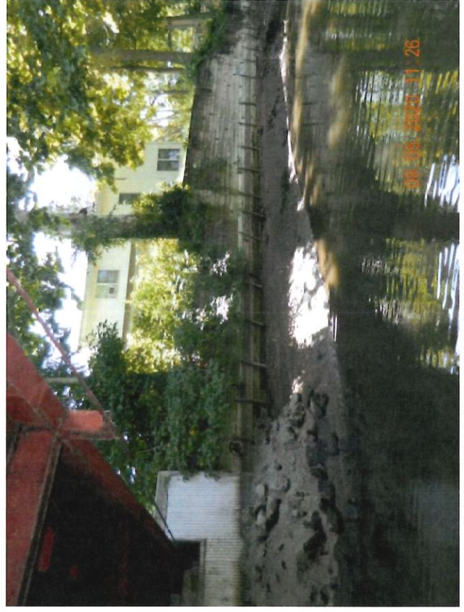
SOUTHEAST RETAINING WALL LEANING
