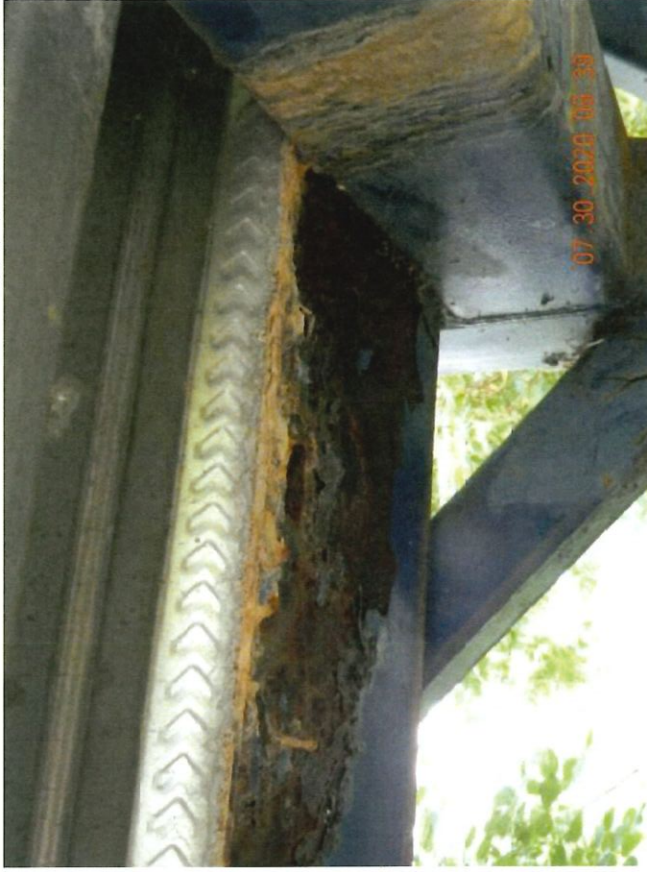
TYP. LEACHING AND RUST AT TRUSS/ DECK INTERFACE
