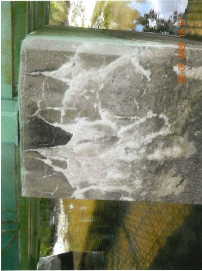
TYPICAL CRACKING WITH LEACHING AT PIERS
