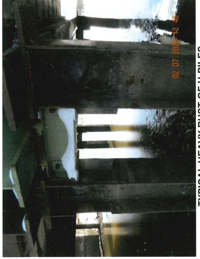
TYPICAL HEAVY RUST OF H-PILES
