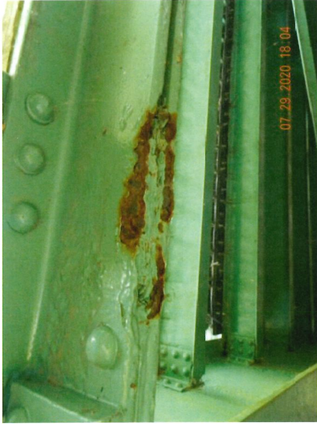
TYP. PACK RUST AT LOWER CHORD OF TRUSS
