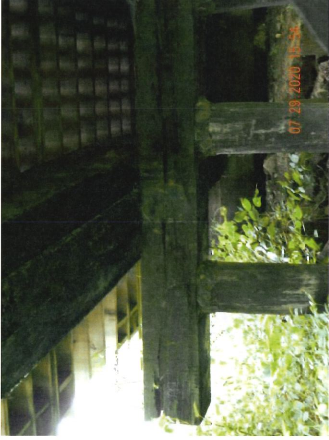
TYPICAL SPLITS IN PIER CAPS OF APPROACH SPANS
