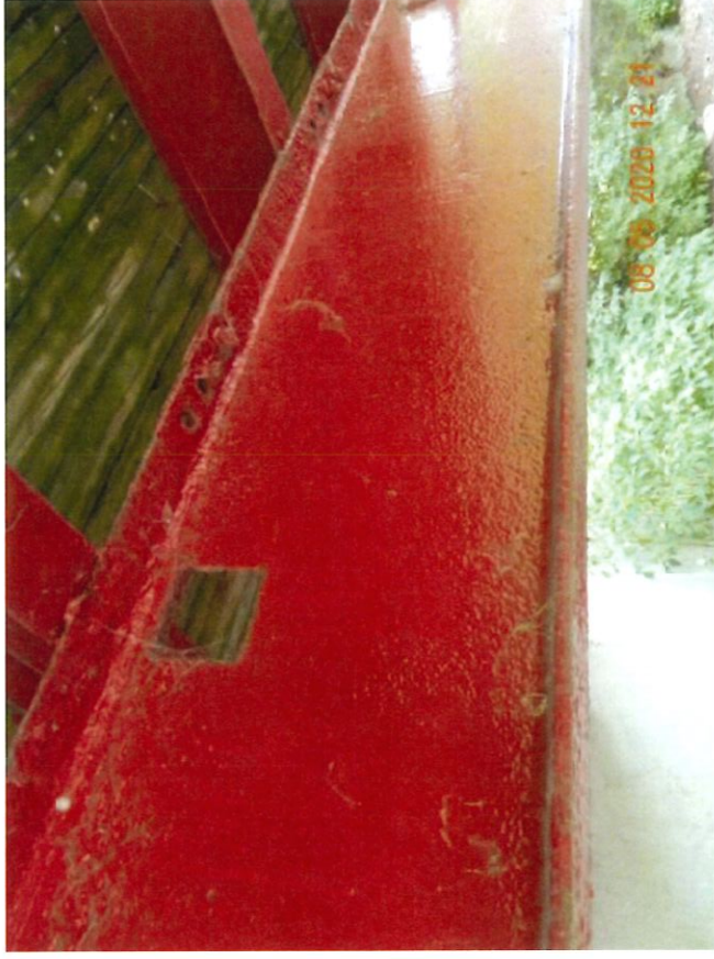
TYP. PITTING OF FLOORBEAMS
