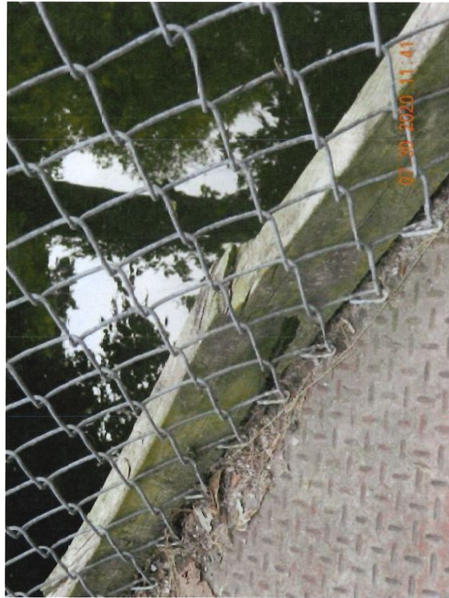
DAMAGED KICKBOARD IN SOUTH RAIL NEAR MIDSPAN
