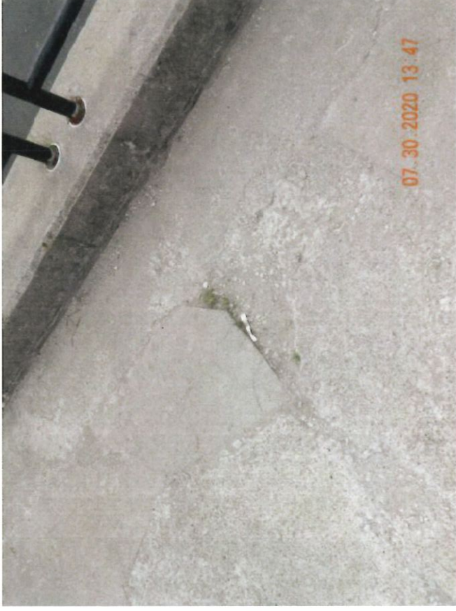
CRACKING AND SCALING IN DECK SURFACE
