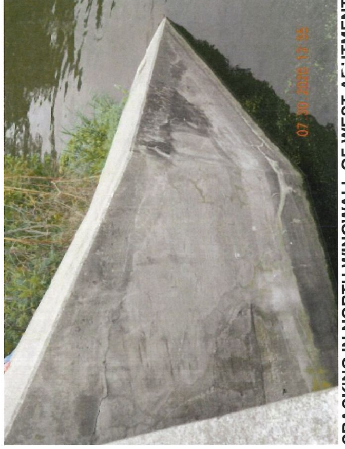
CRACKING IN NORTH WINGWALL OF WEST ABUTMENT
