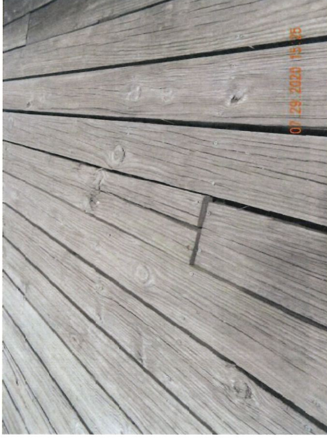
SPLITTING OF TIMBER DECK BOARDS
