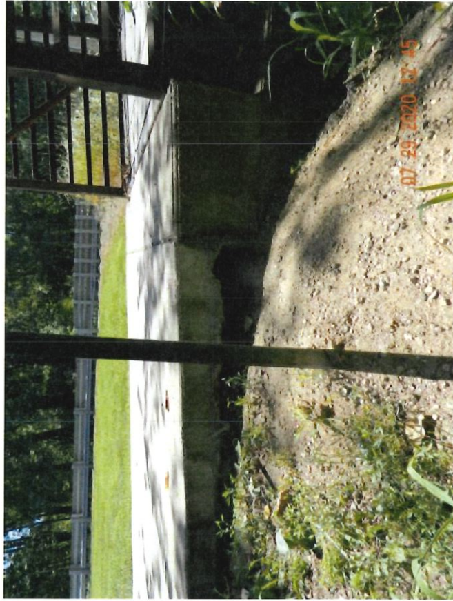
UNDERMINING AT EAST APPROACH
