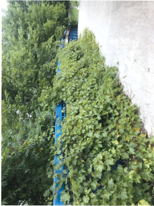
HEAVY VEGETATION ON WEST TRUSS
