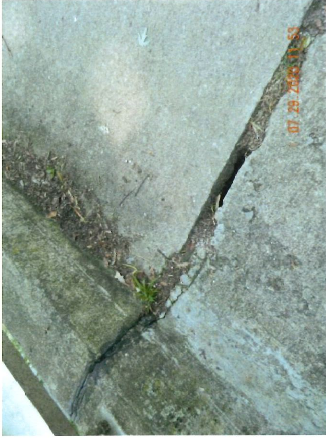
FAILED EAST EXPANSION JOINT DECK
