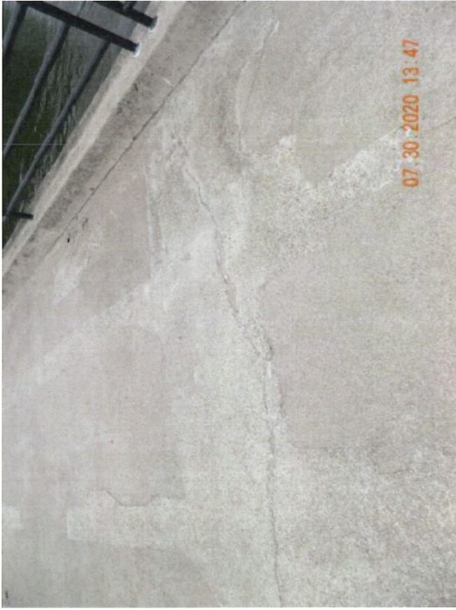
TYP. CRACKING IN DECK SURFACE
