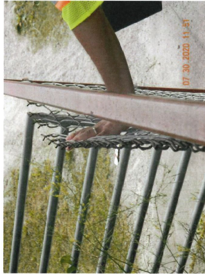
LOOSE FENCE IN NORTH RAIL AT EAST END
