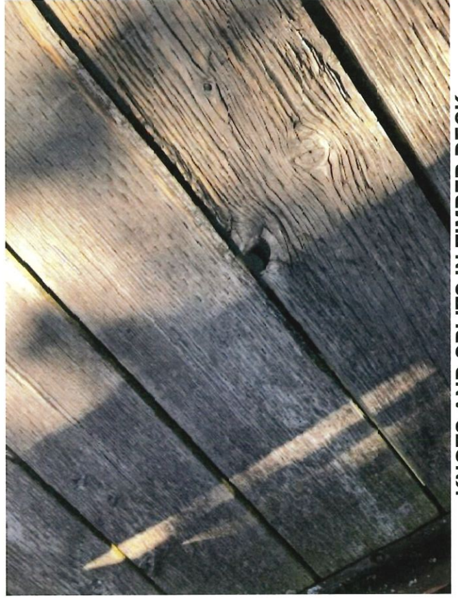
KNOTS AND SPLITS IN TIMBER DECK
