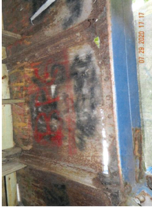
00% SECTION LOSS IN WEB PL OF S. GIRDER AT 3RG.
