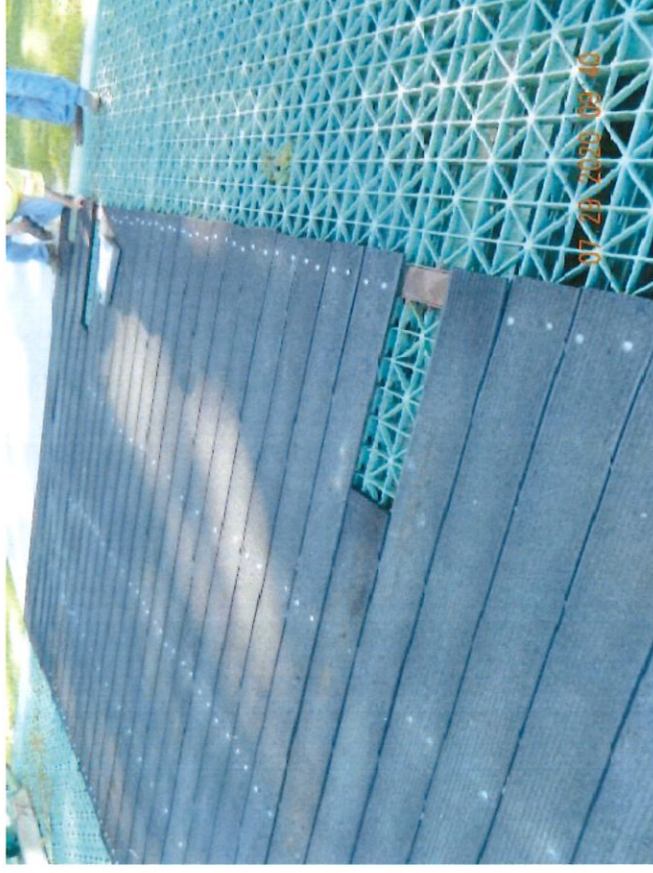
TYP. RUBBER MAT PIECES MISSING
