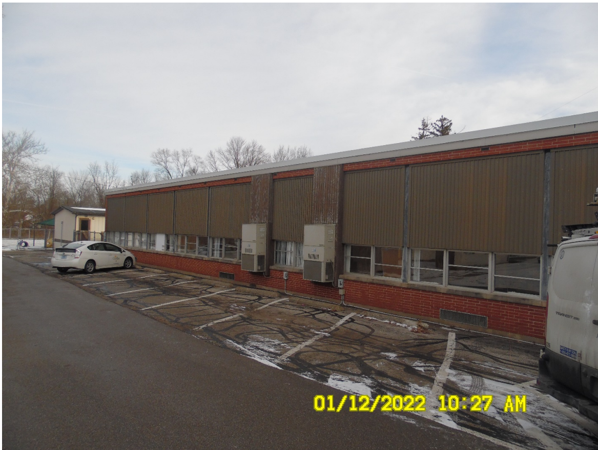
Classrooms on north end of building to be converted to bedrooms and offices for group housing quarters use
