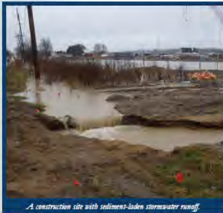
A construction site with sediment-laden stormwater runoff.
