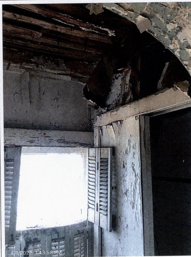
Collapsed ceiling + water damage Front porch entry
