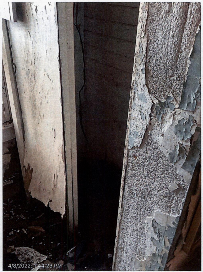
Damage From roof leak
