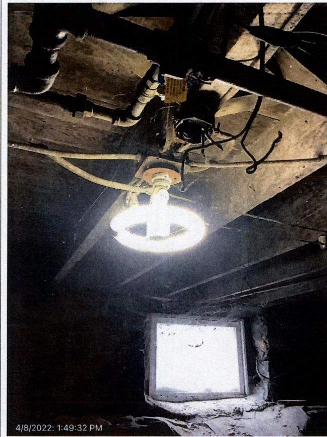
New light Fixture / old wires exposed
