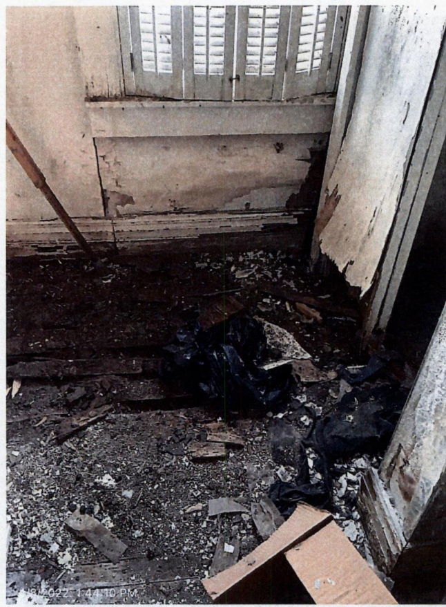
Damage from roof leak Front Porch entry
