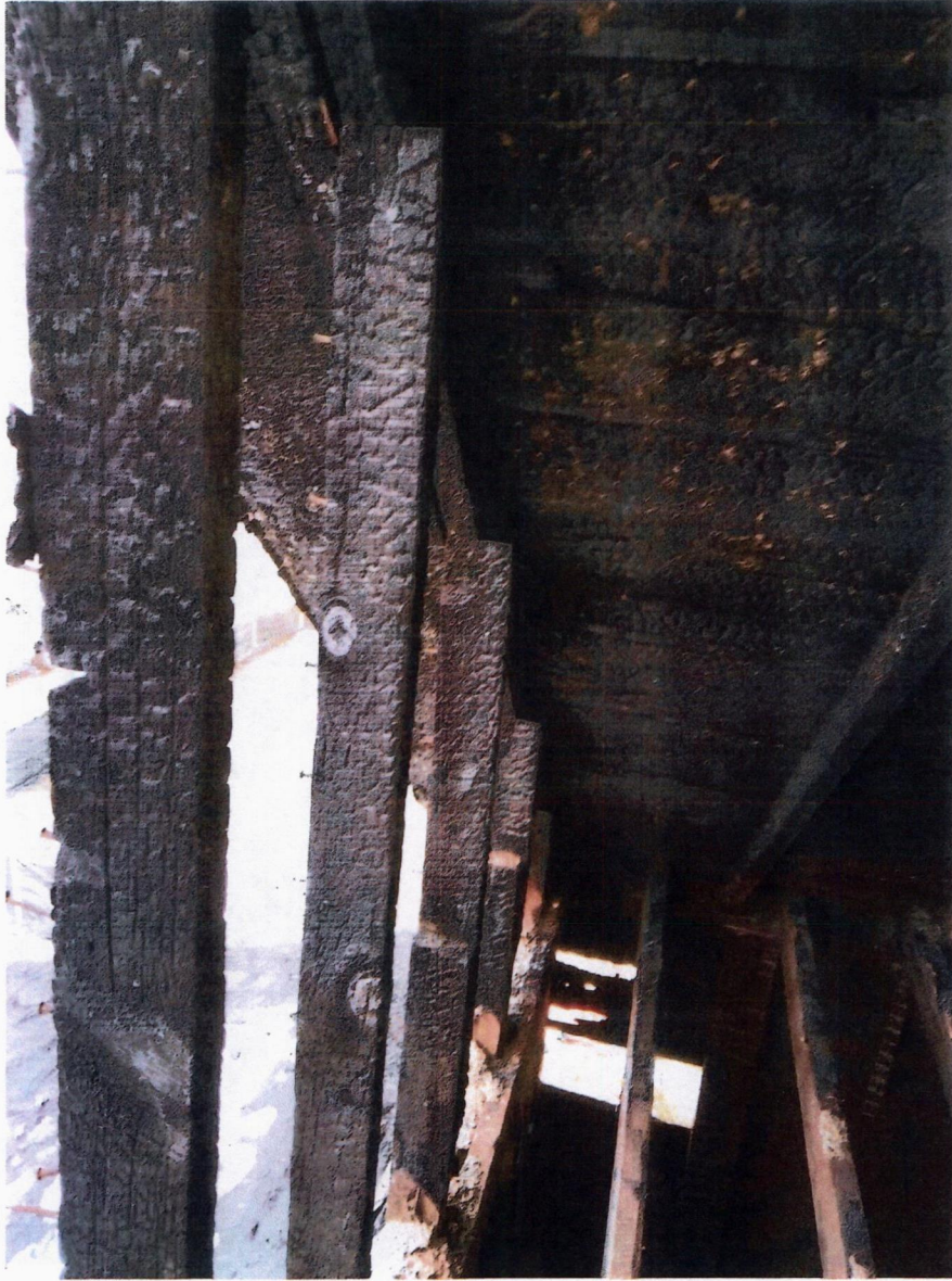
Front Wall Damage
