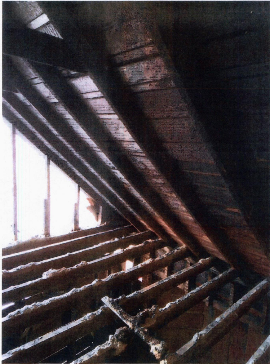
Sheathing more smoke damage than structural
