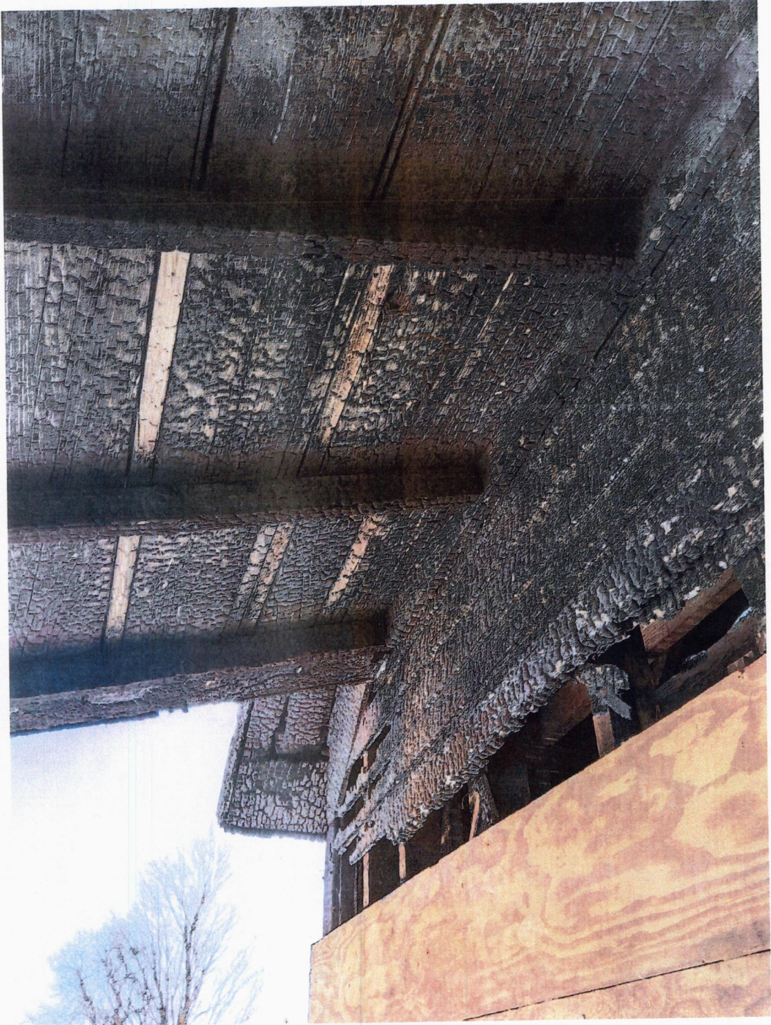
Porch Roof Damage
