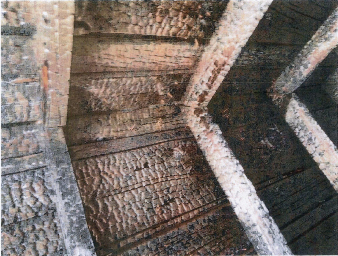
Sheathing damage at top 2'-0" front section
