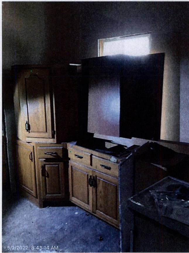
Cabinet never installed
