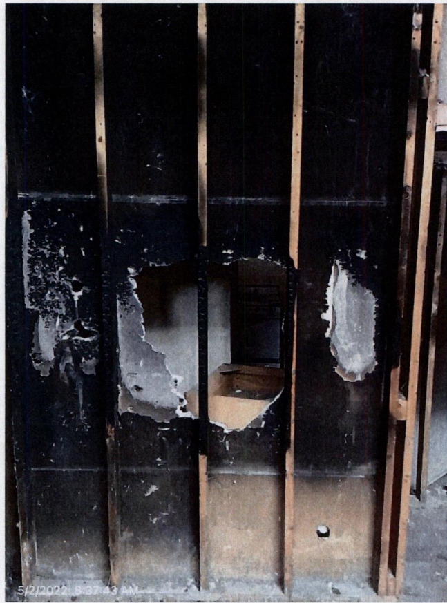
Charred 2x4 Wall Beams
