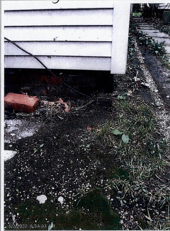
missing bricks corner of foundation
