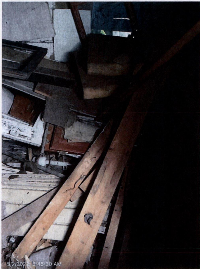
Debris in basement
