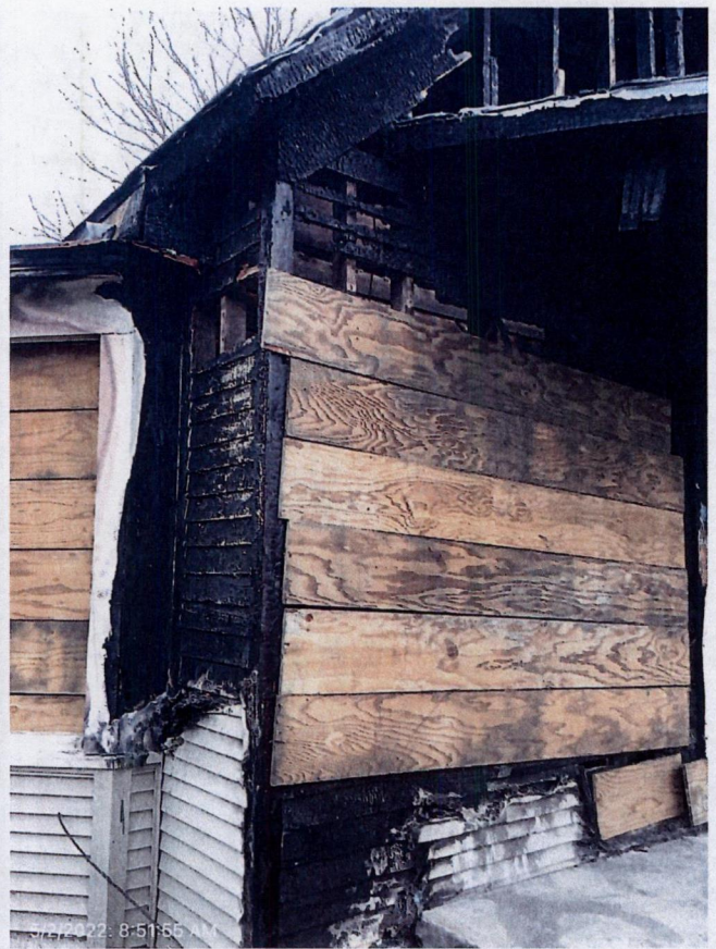
Front porch fire damage
