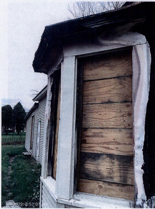
Siding damage Window damage
