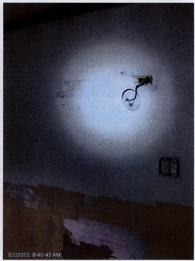
loose exposed wires
