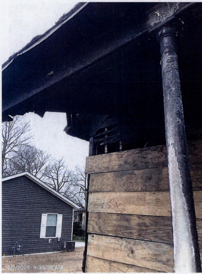
front porch fire damage
