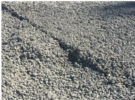
7 CRACKING & 15 RAVELING (POOR)
