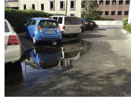
6 PONDING / STANDING WATER
