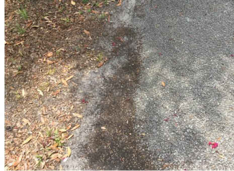
5 UNSTABLE DRAINAGE AREA & 14 DEBRIS (MARGINAL)
