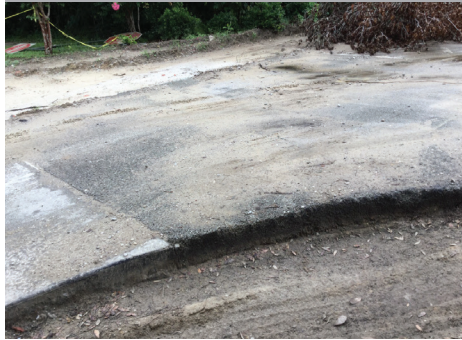
5 UNSTABLE DRAINAGE AREA & 13 SEDIMENT (POOR)
