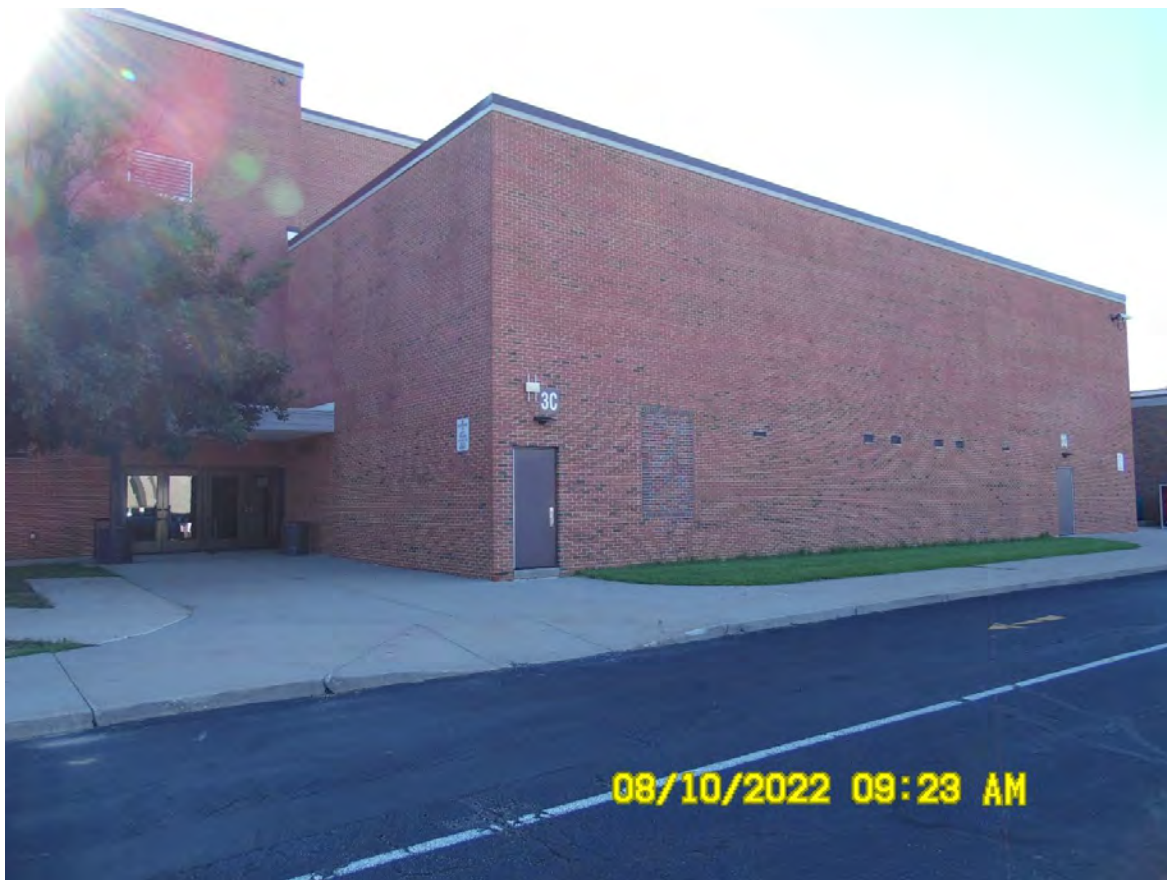
Looking southeast at wall on which the proposed sign will be installed
