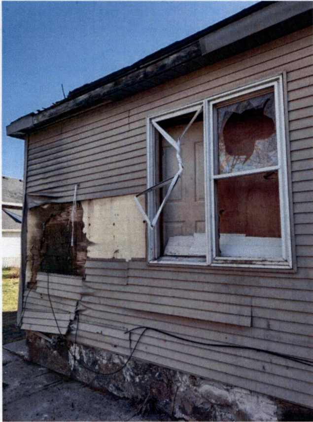
Fire damage at rear of property.
