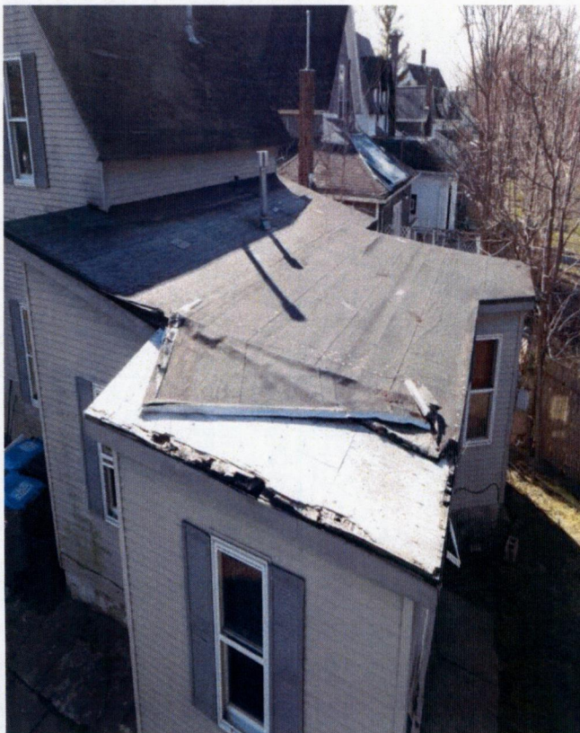
Damaged roof at rear of property
