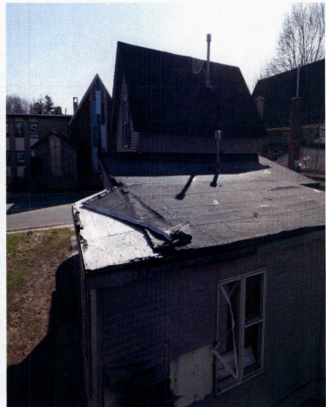
Damaged roof at rear of property.
