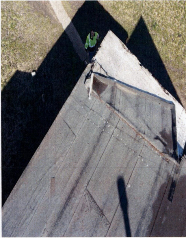
Damaged roof at rear of property.
