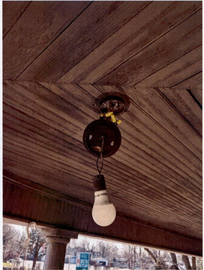
Exposed exterior wiring.
