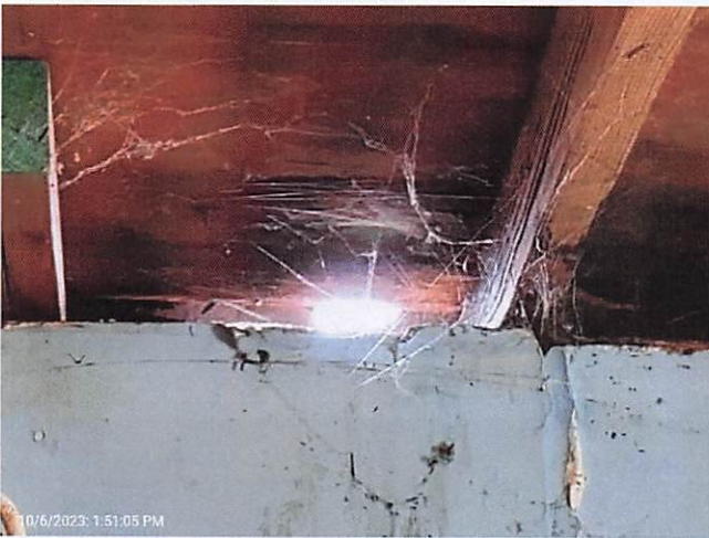
10/6/2023: 1:51:05 PM Hole in roof in rear entryway.
