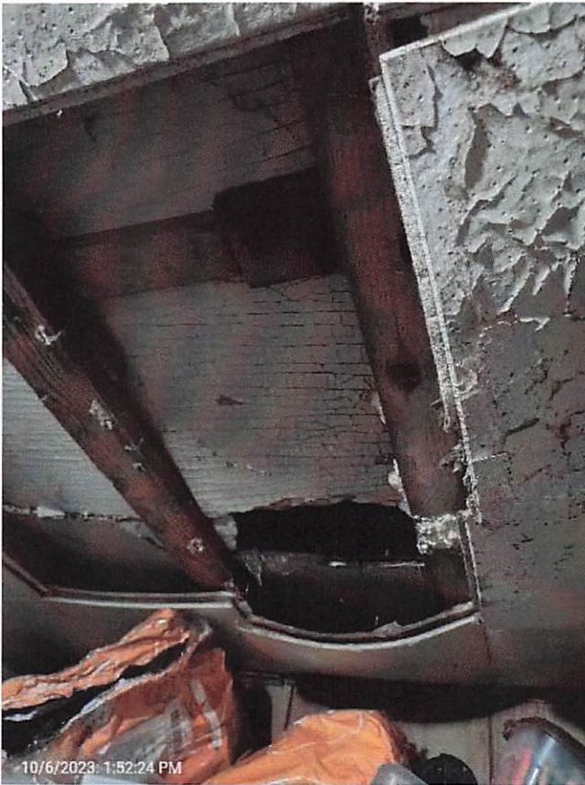
Damaged ceiling in bedroom.
