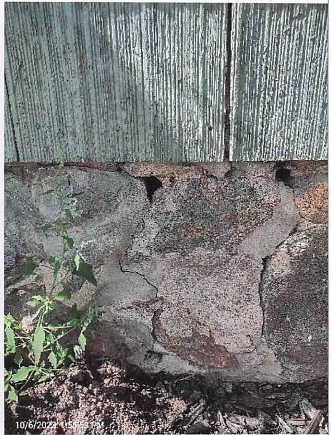
Gaps in foundation.
