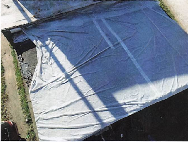
Plastic covering roof at rear of property.
