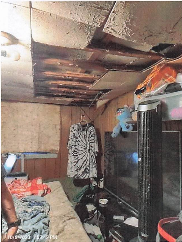
Damaged ceiling in bedroom.
