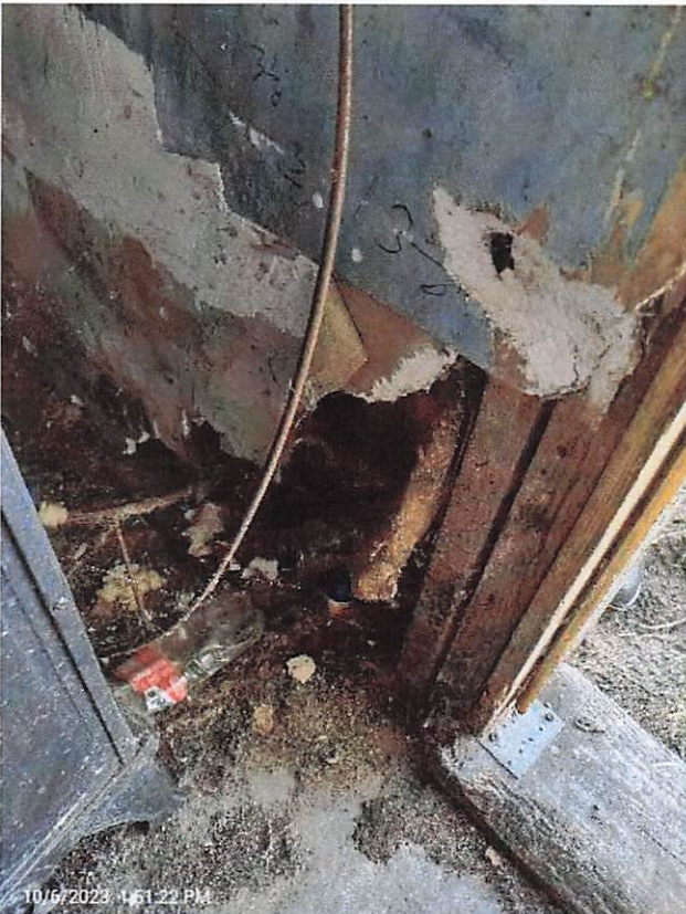
Damaged wall near back door.
