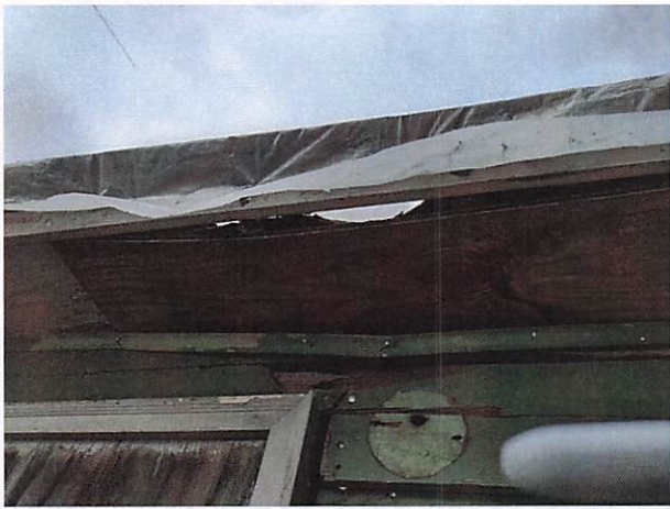
Damaged fascia at rear of property.
