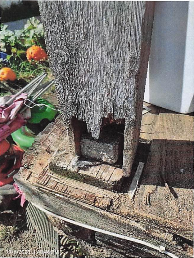
Damaged support post on porch.
