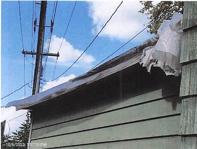
Plastic covering roof at rear of property.
