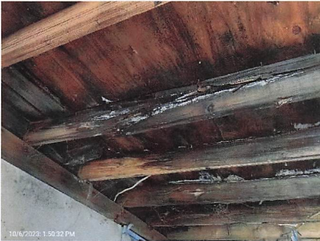
10/6/2023: 1:50:32 PM Water damaged roof support.
