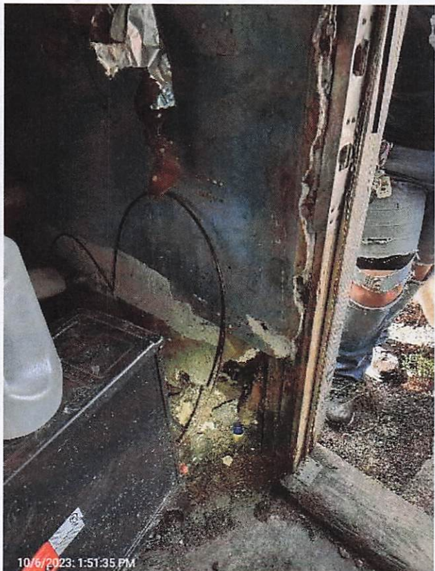
Damaged wall near back door.
