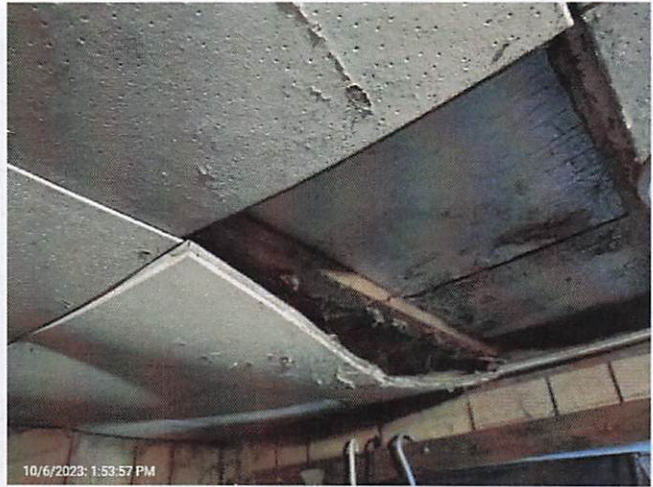
Damaged ceiling in bedroom.
