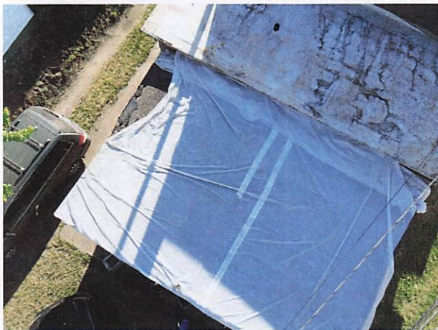
Plastic covering roof at rear of property.
