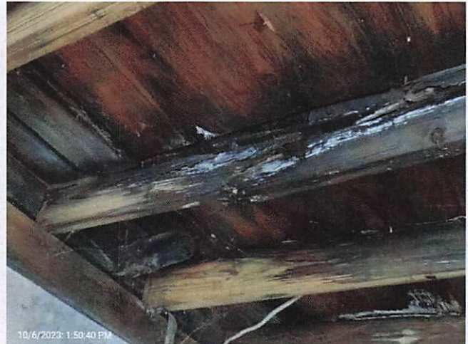
10/6/2023: 1:50:40 PM Water damaged roof support.
