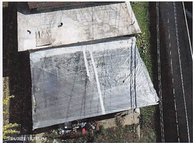
Plastic covering roof at rear of property.
