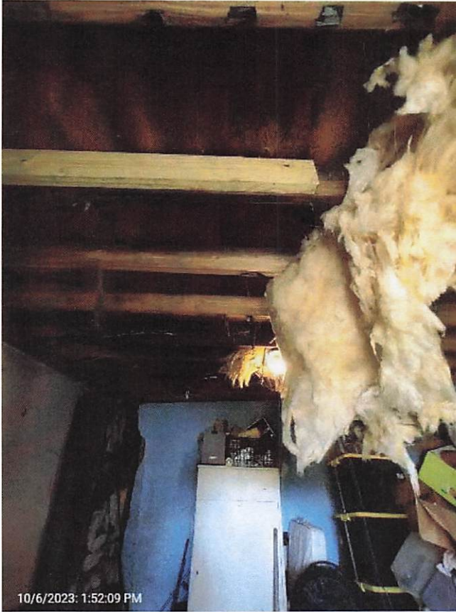
Damaged ceiling at rear of property.
