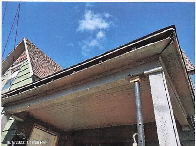
Temporary post added to provide support on porch.
