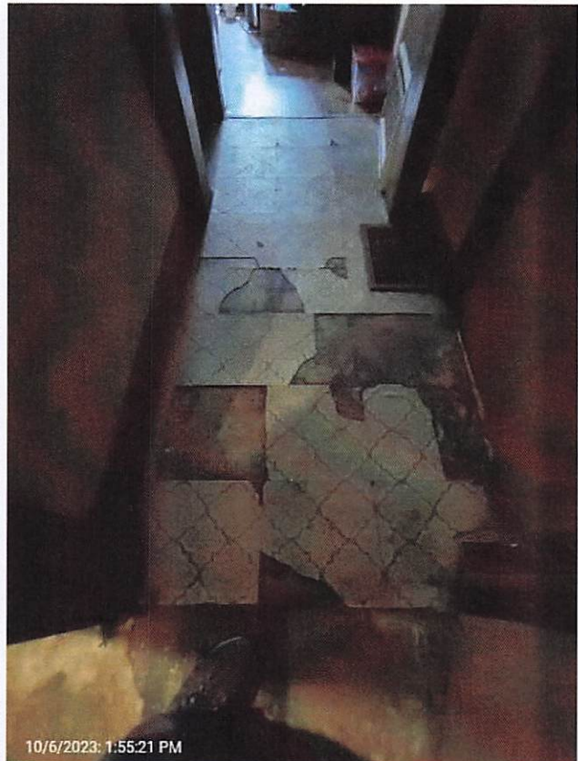
10/6/2023: 1:55:21 PM Damaged floor coverings in hallway near bathroom.
