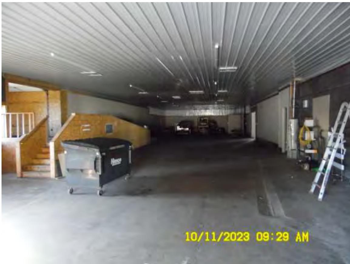
Bay in northeast corner of building proposed as wash area. Trench drain pictured on lower right.
